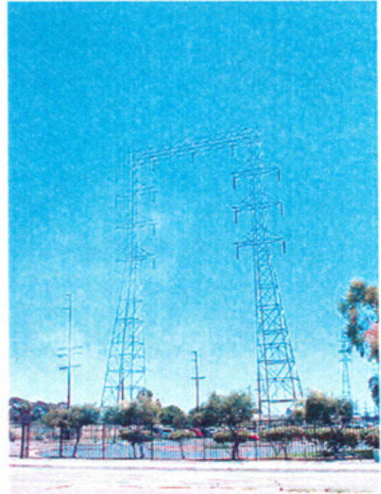
Photo 3: Tower 10, Corner of Lagoon Drive and F Street
