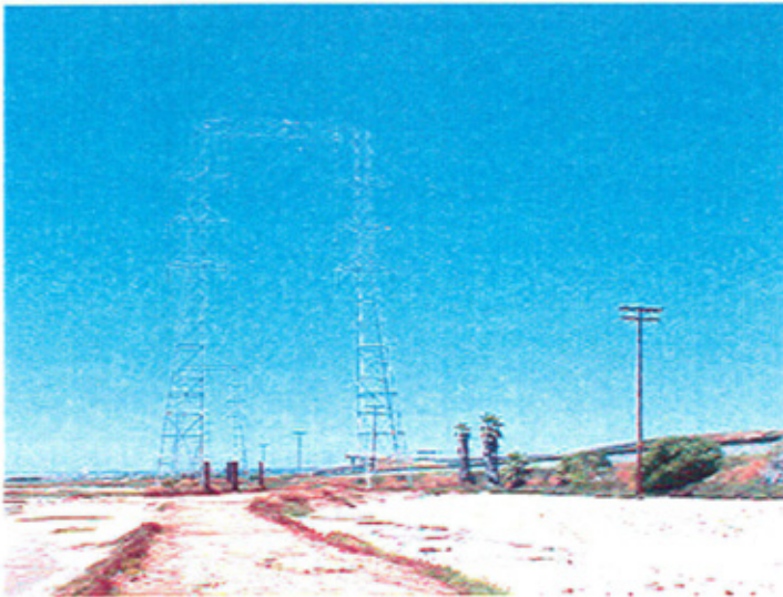
Photo 6: Tower 15, Looking Northwest in Sweetwater Estuary
