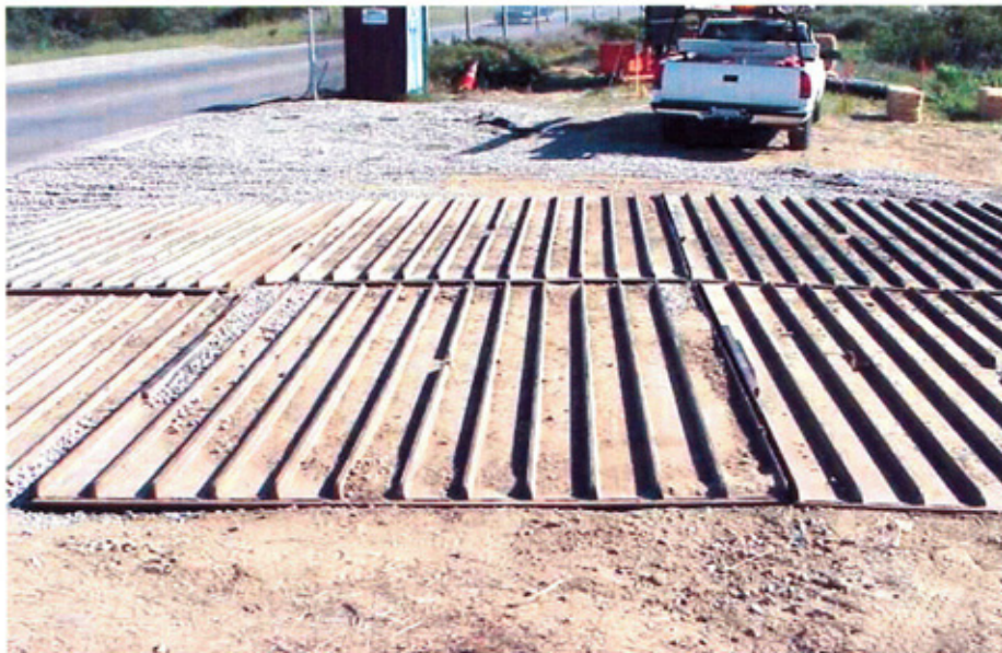
Manufactured metal plates knock dirt off vehicles before exiting a site.
