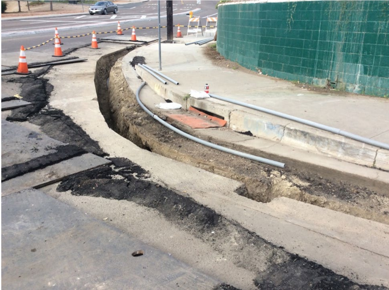
Figure 8: Trenching Work for Electrical Power Supply Installation at the Massachusetts and Main Site
