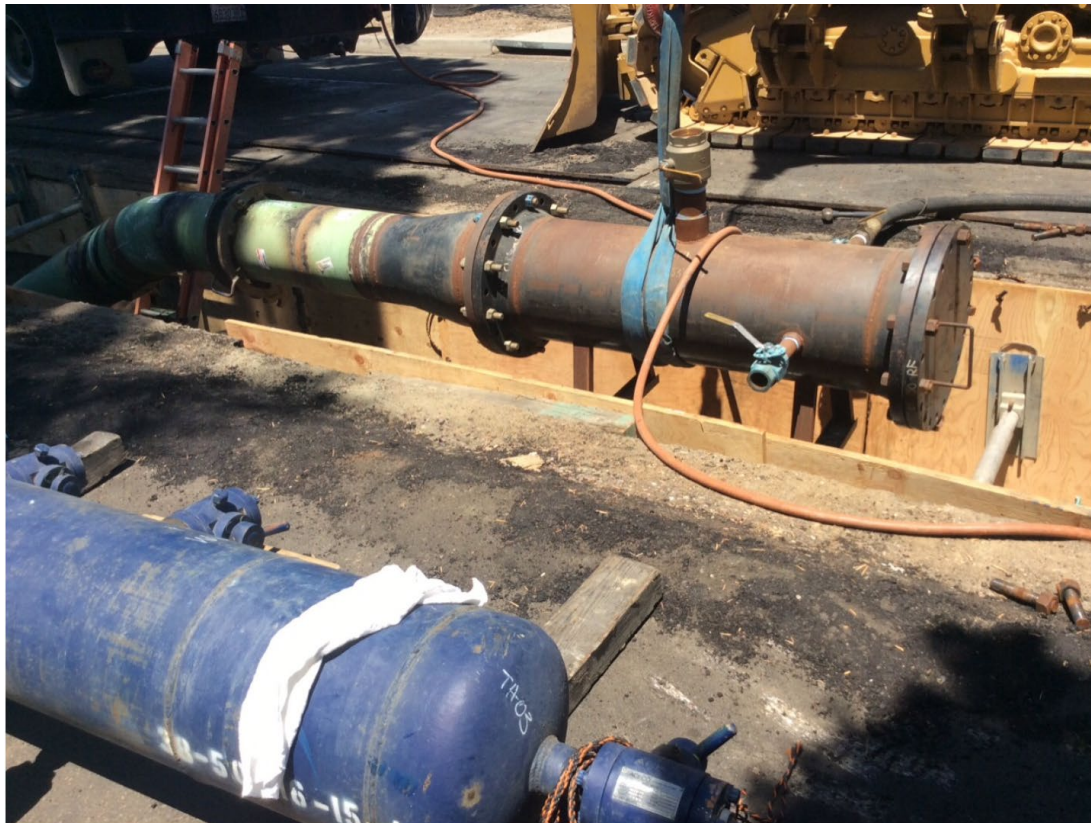
Figure 6: Section 6 Test Head in the Foreground, Temporary Pigging Equipment in the Background
