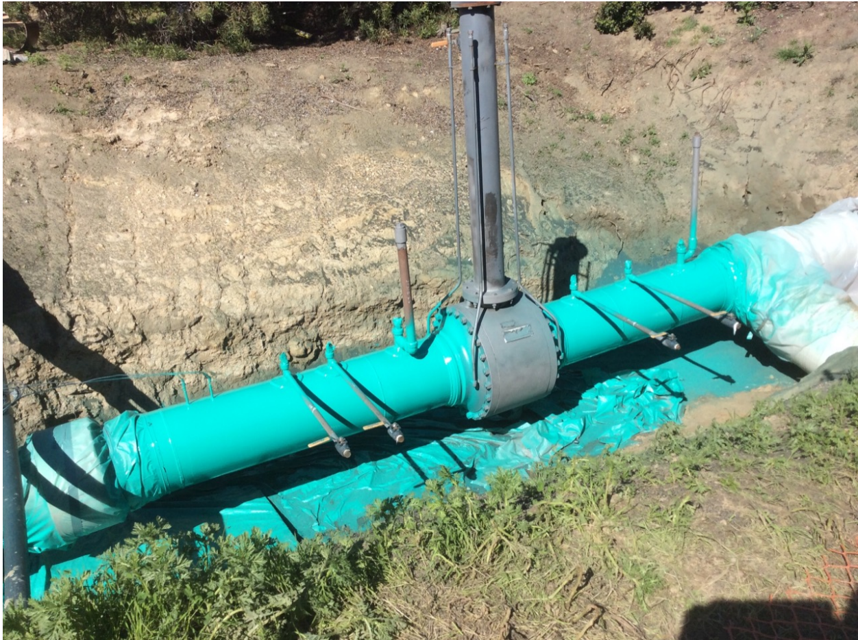
Figure 3: Mainline Valve Assembly With Instrument Piping
