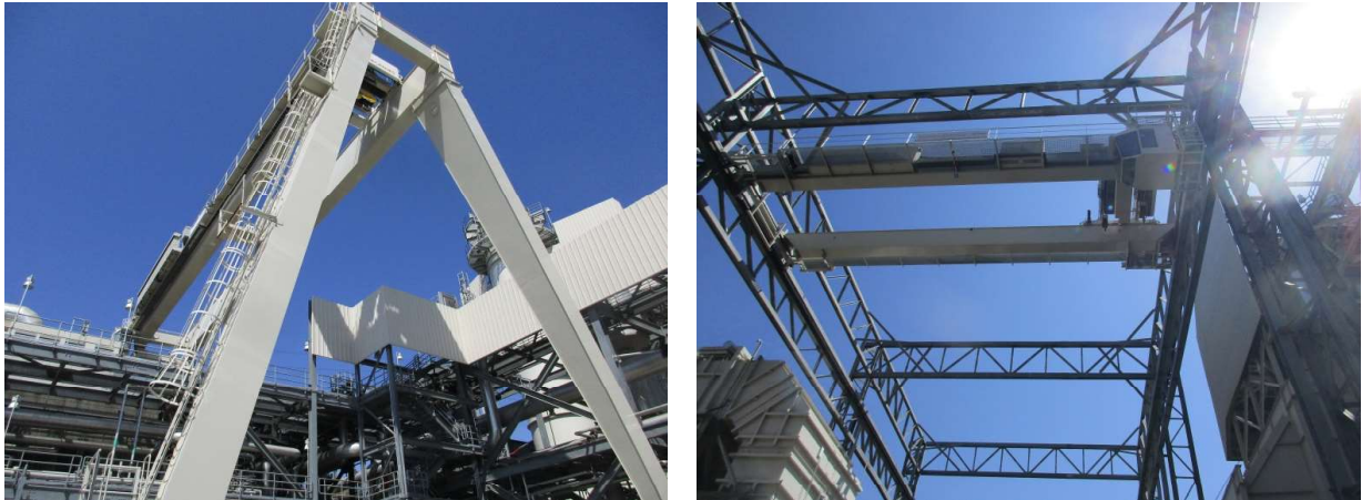
Figure 5-4 — Palomar Cranes Installed in 2014
