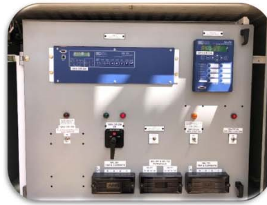
Digital Relay Equipment
