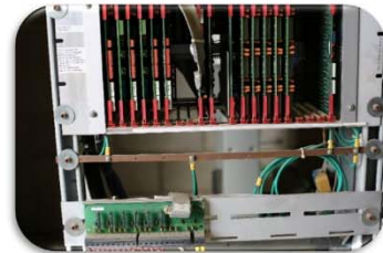
Aging Remote Terminal Units
