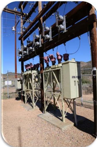
Oil Circuit Breakers
