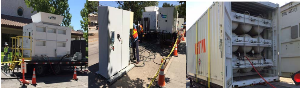
Figure 3: CNG Capture portable generator, mobile compressor, and CNG trailer 49
