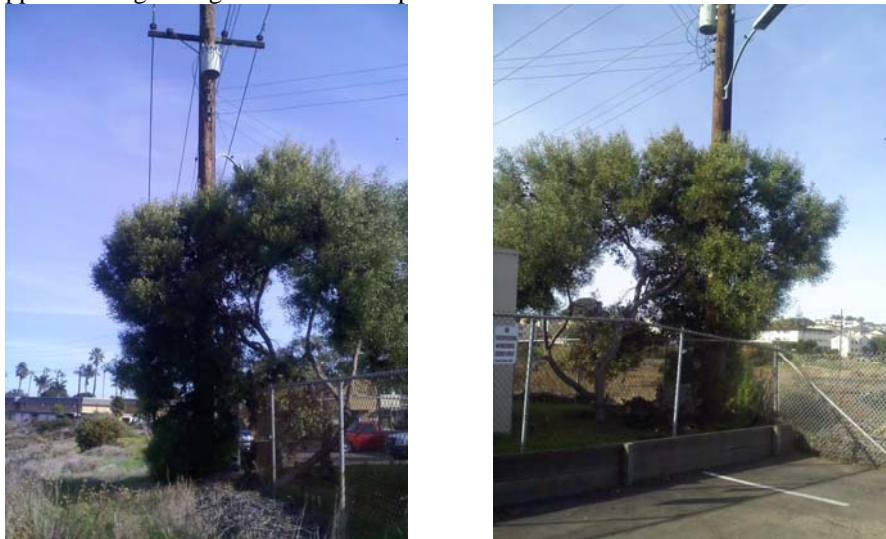
Example: From one side of the pole it appears to need trimming for climbing space. But the proximity to the parking lot allows bucket access negating the climbing access issue.
