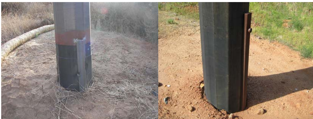
Example: Exempt above grade ground wire covers. These poles do not require brushing.
