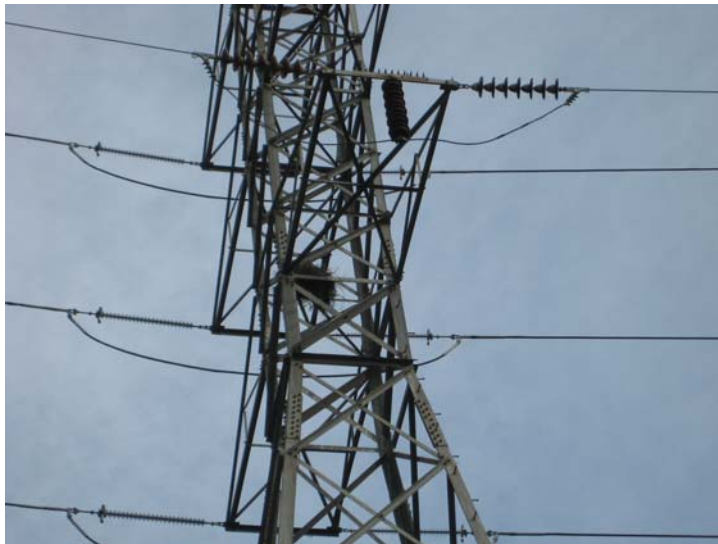
Example: Raptor nest in a steel transmission tower near Mission Valley
