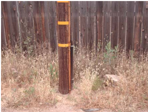
P277890 has lots of dry grasses at the base of the pole and would require brushing in SRA.
