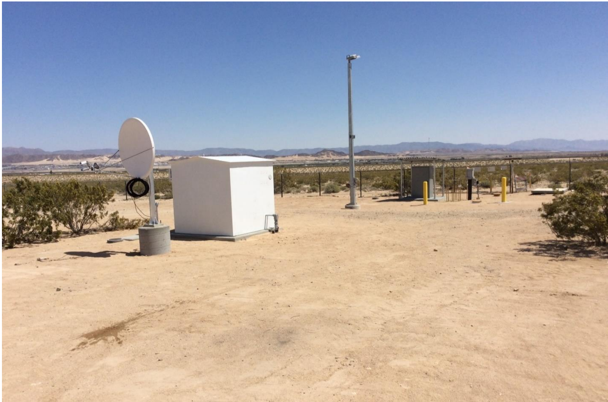
Figure 6: Indian Trail – Satellite Communications Equipment and Electrical Shelter in Foreground, Linebreak Cabinet and Actuator in Background
