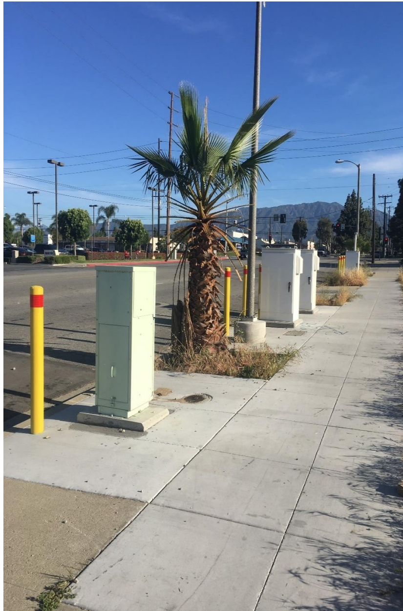
Figure 4: Cabinets for Automation
