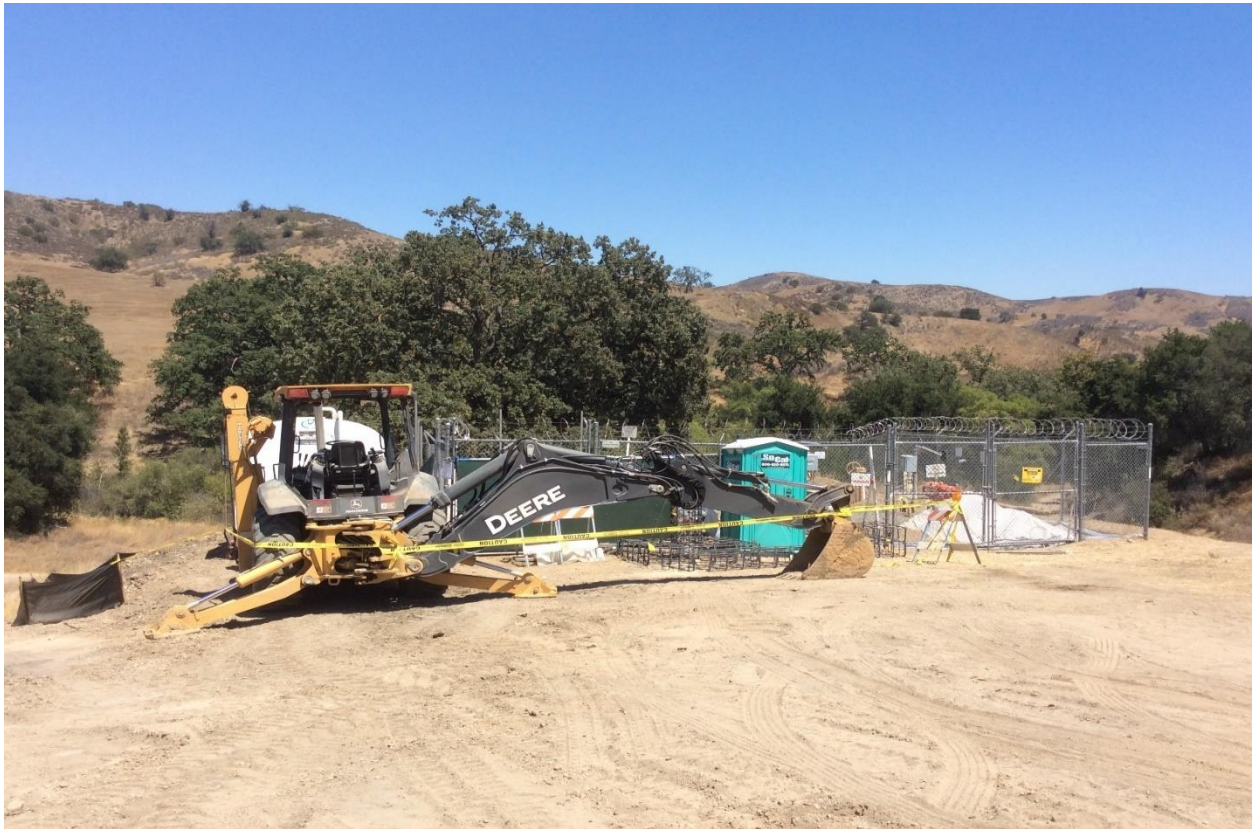
Figure 9: Equipment at Simi Tap
