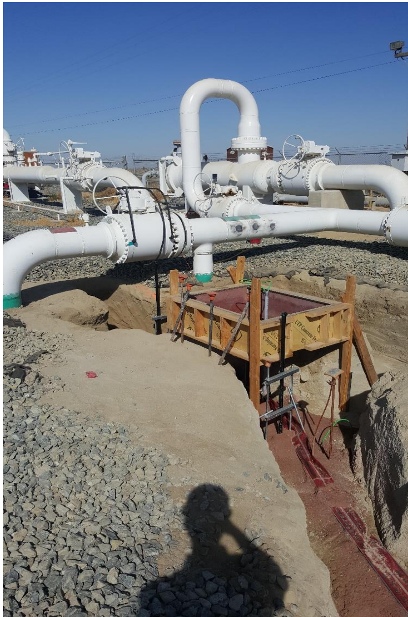
Figure 5: Delano Site Excavation for New Linebreak Cabinet in Foreground, Existing Piping Configuration in Background
