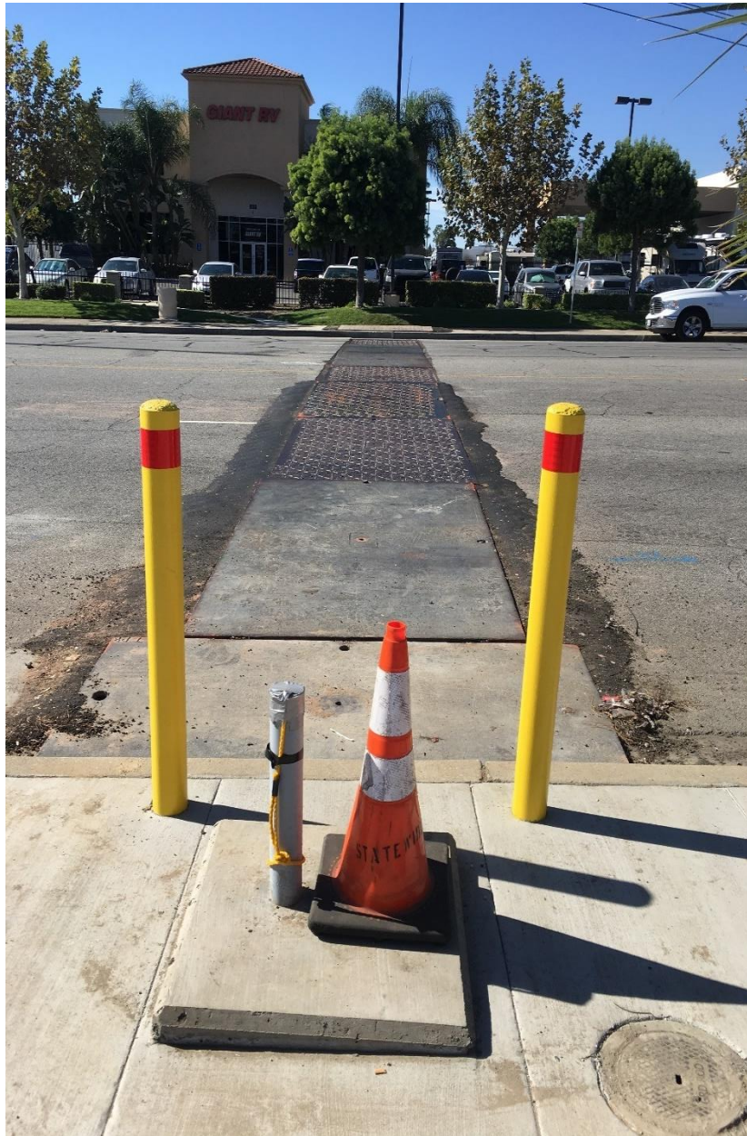
Figure 3: Underground Power Crossing Benson Avenue
