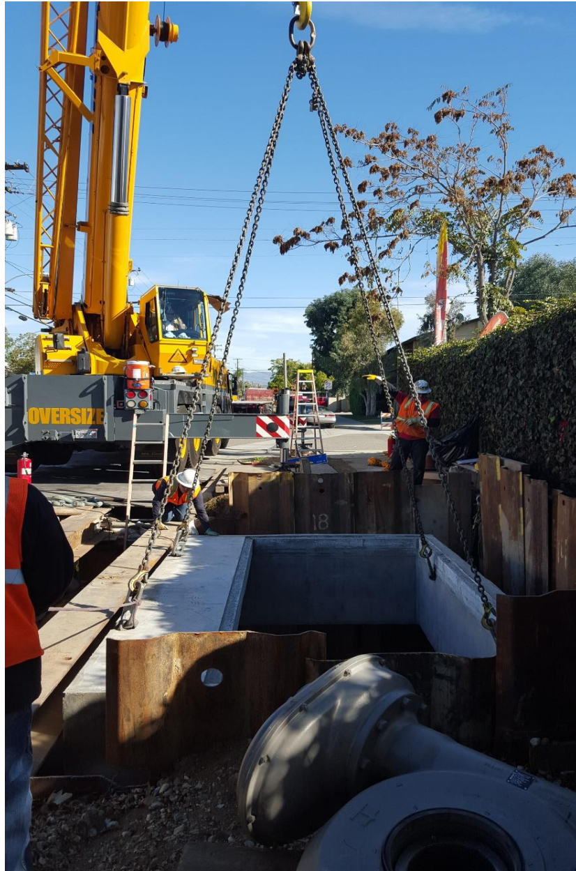
Figure 5: Orange Valve Enhancement Project Bundle, Walnut and Cypress Site – Placement of the Vault
