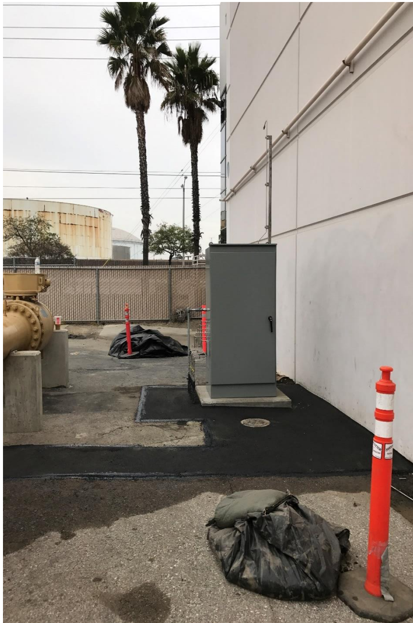
Figure 5: New Linebreak Panel to Monitor the Pressure of Line 325 for Automatic Closure
