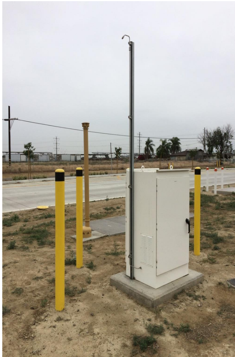
Figure 2: Instrument Cabinet in Foreground: Vault Lid and Vault Vent in Background – Post Construction
