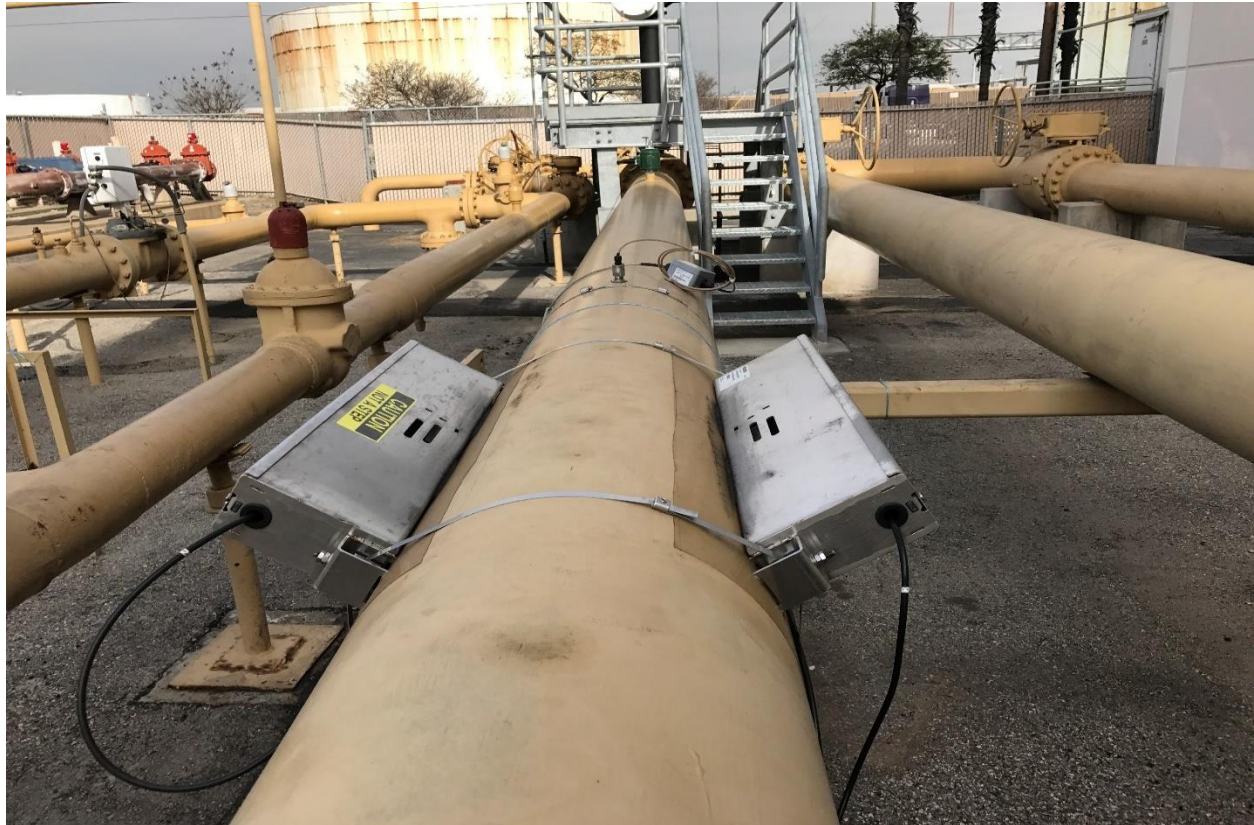
Figure 4: Ultrasonic Flow Meter Installed on Line 325
