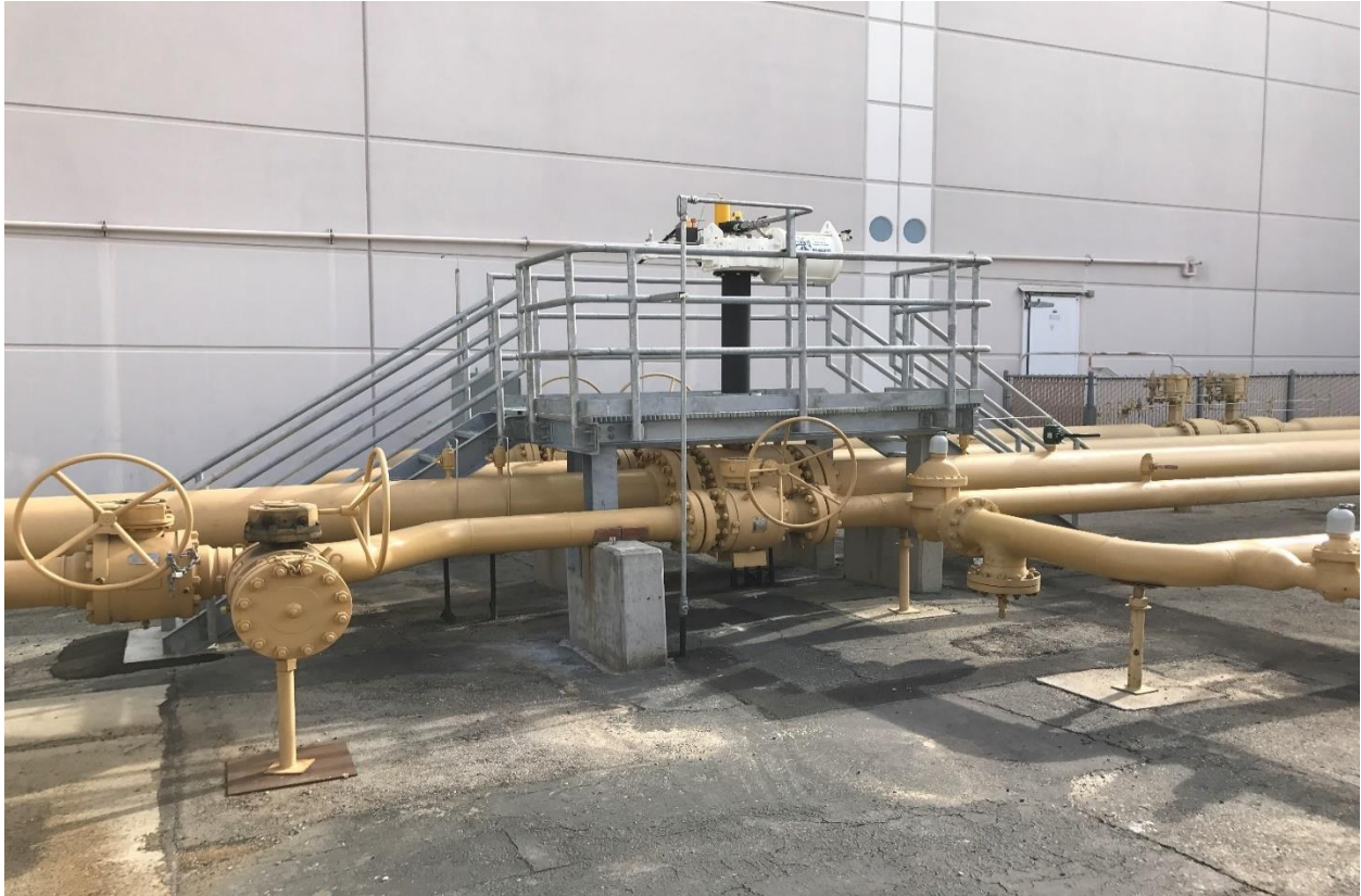
Figure 3: New Actuator and Platform for Maintenance and Operations
