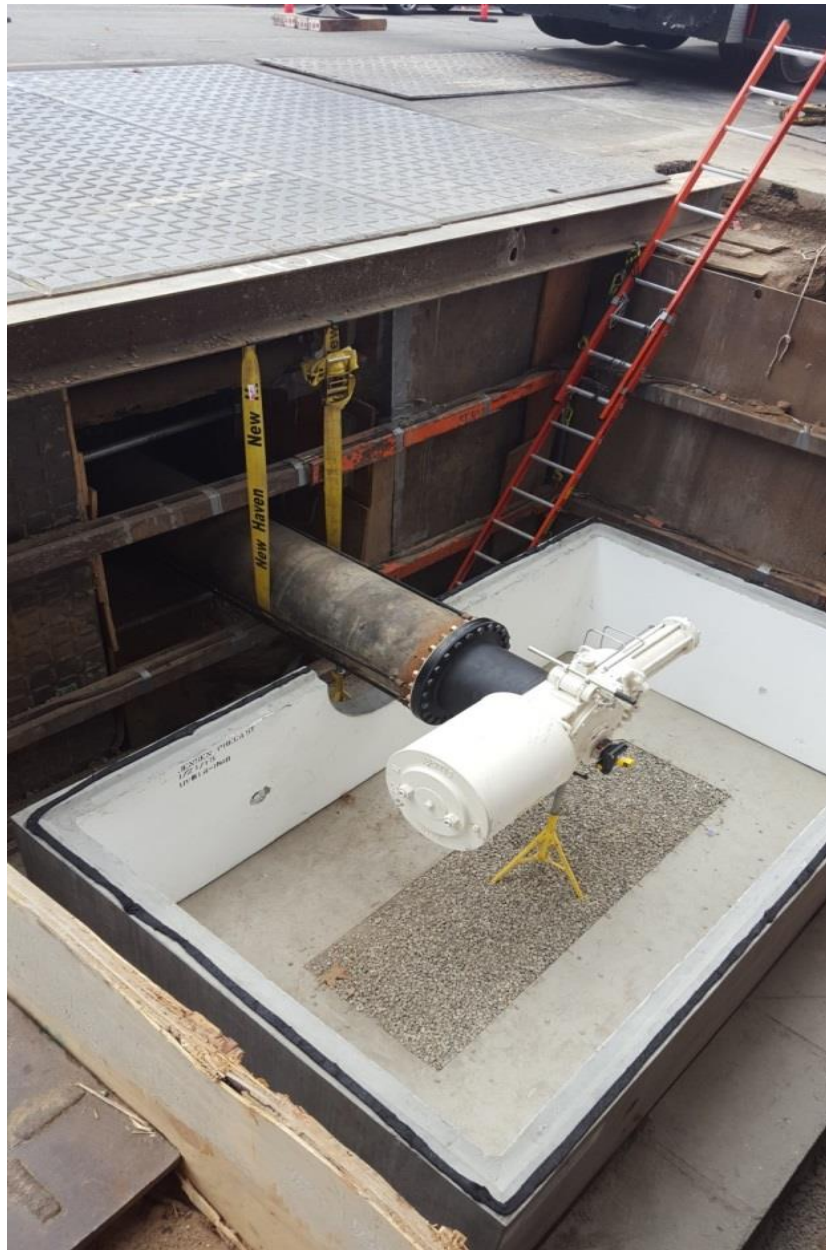
Figure 7: Orange Valve Enhancement Project Bundle, Almond and Citrus Site –Bottom Section of the New Vault and Actuator
