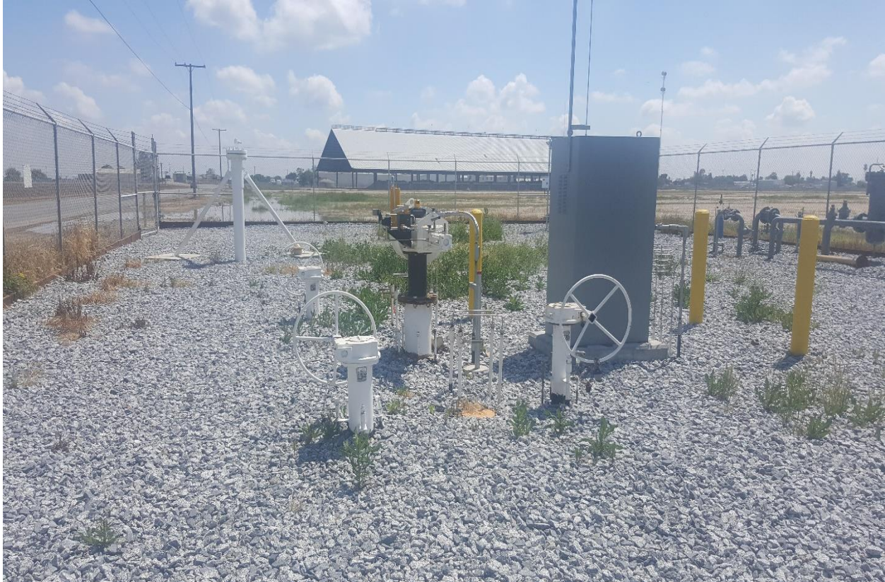
Figure 6: Tipton Site New Actuator and Linebreak Cabinet in Foreground, Blowdown in Background
