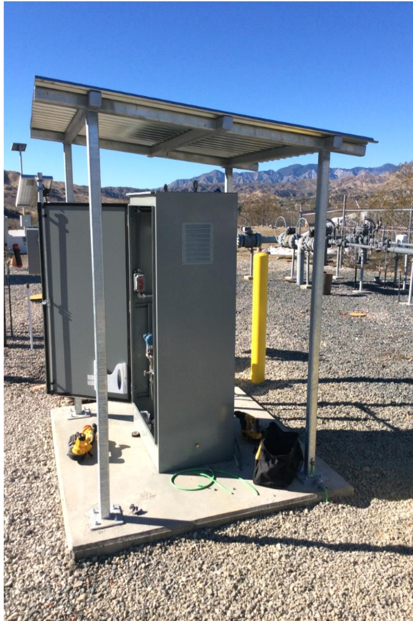
Figure 7: Malibu Trail – Linebreak Cabinet and Canopy
