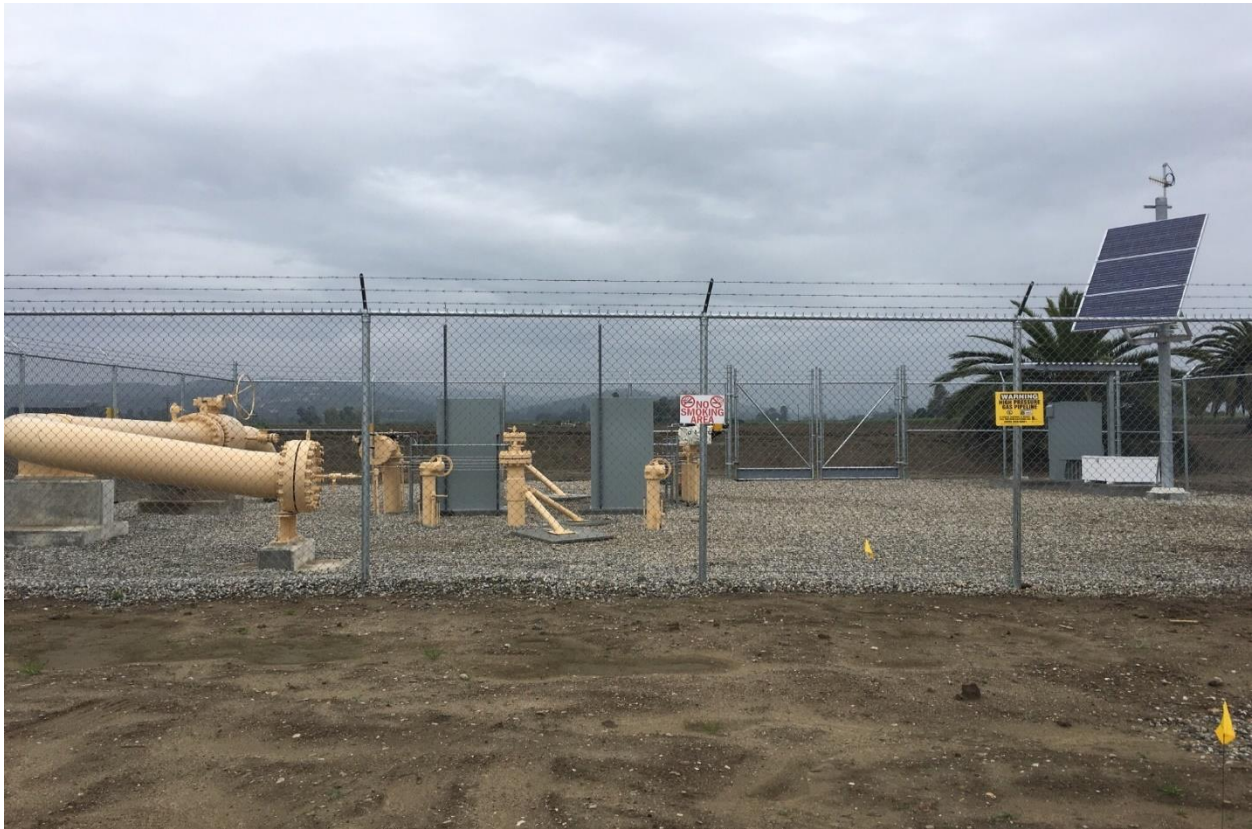
Figure 6: New Cabinets and Solar Panel at Santa Clara West
