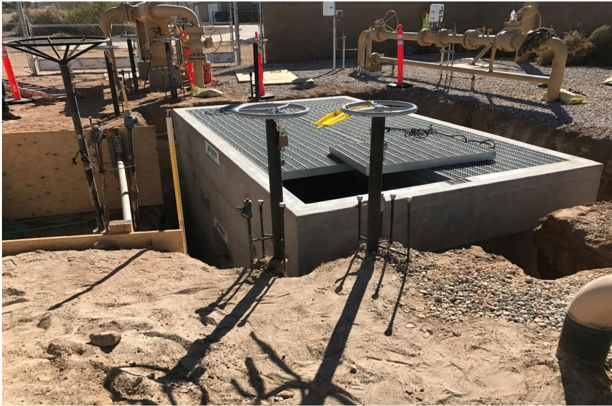
Figure 3: New Vault in the Foreground, Existing Piping in the Background
