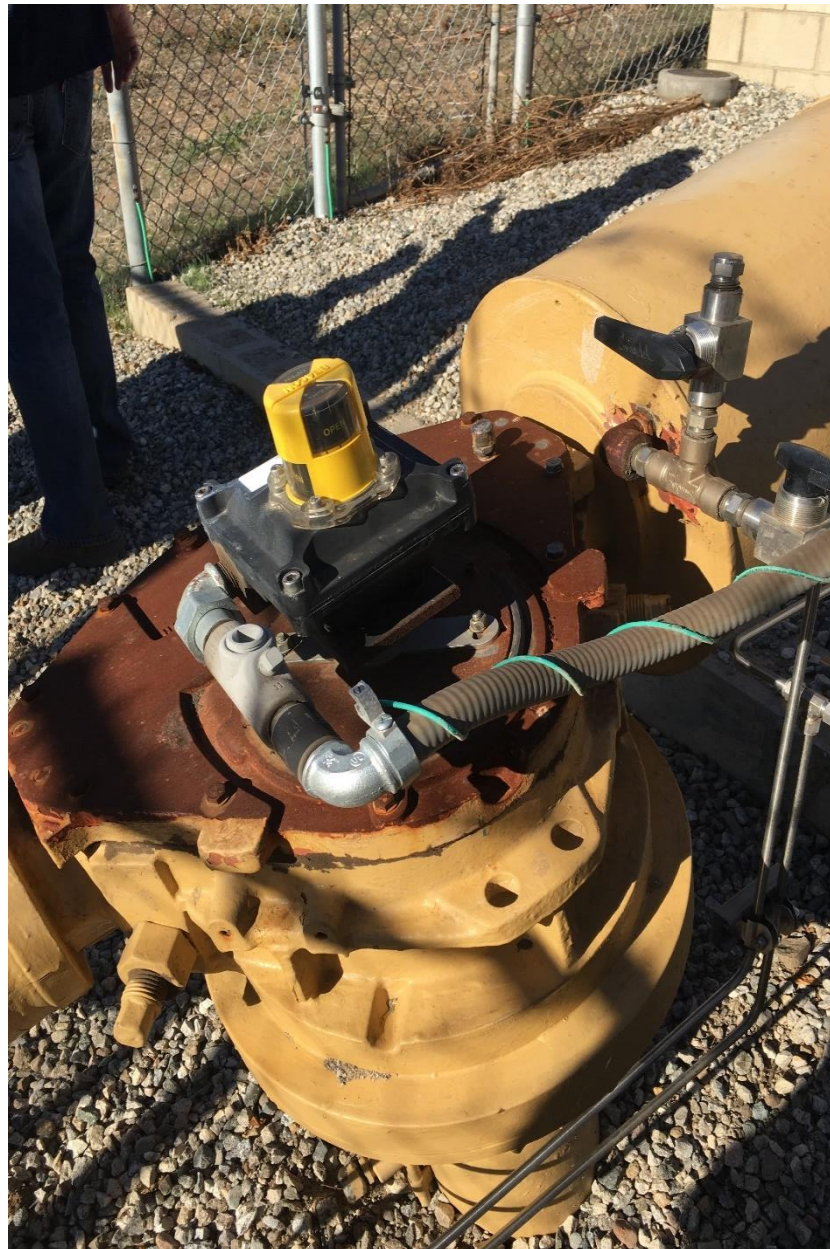
Figure 5: New Position Indicator at Hall Canyon
