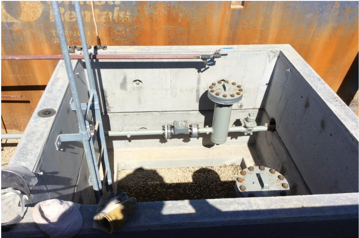
Figure 6: Regulator Station Vault
