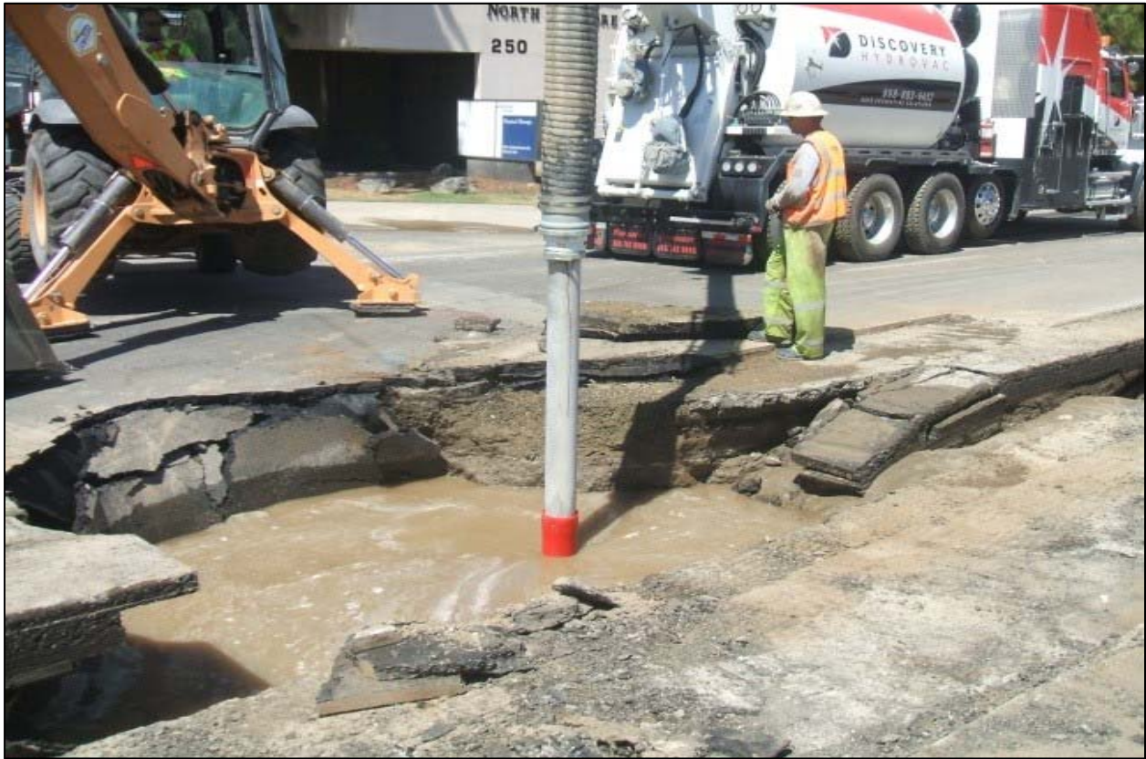
Figure 6: Section 2 - Broken Waterline Clean Up
