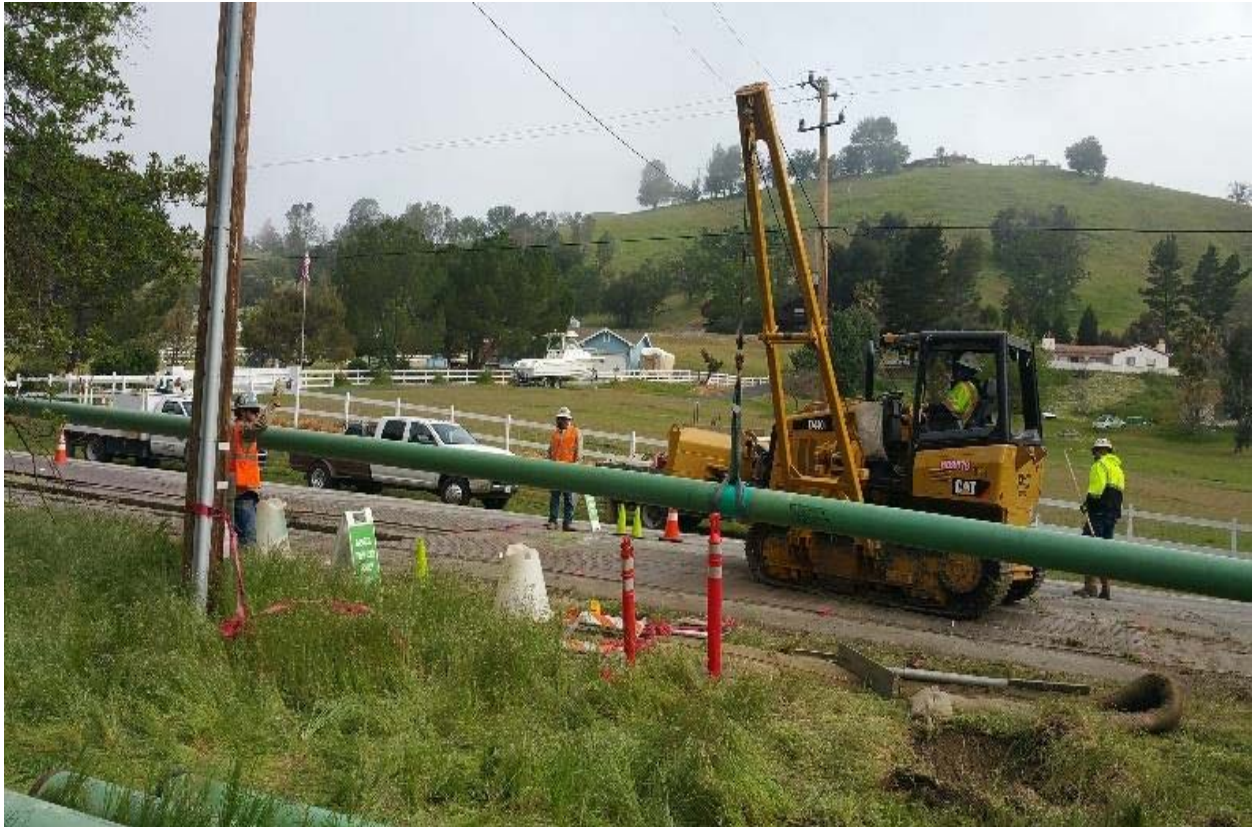
Figure 4: Spotter Signaling to Operator Overhead Wires
