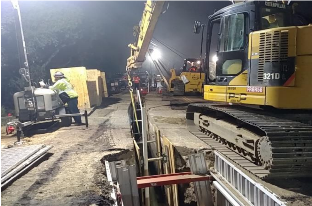
Figure 15: Section 7B - Shoring and Placement Equipment Used to Maintain Integrity of the Excavated Trench
