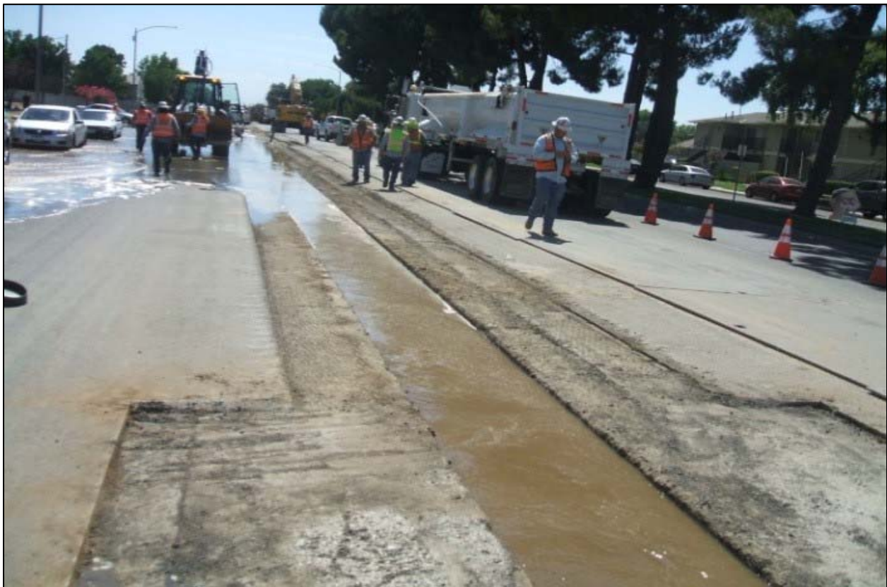
Figure 5: Section 2 - Broken Waterline
