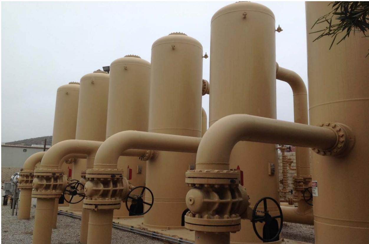
Figure 5: Existing Obsolete Equipment
