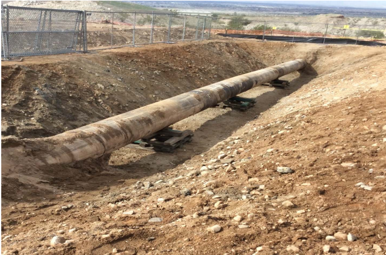
Figure 9: Temporary Pipe Supports (TB-7) Under Line 2000 in Preparation for a Test Break
