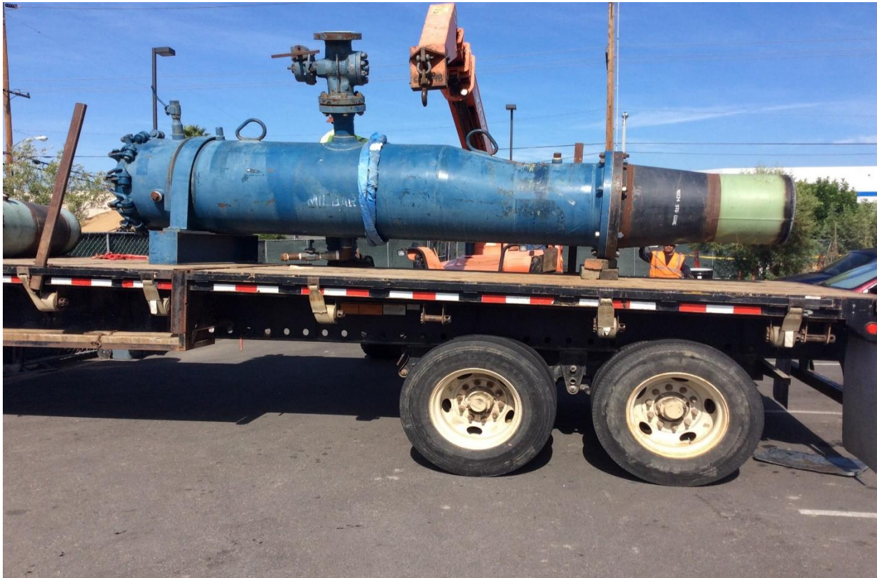
Figure 7: Off-loading Pig Launcher (used for launching multiple pigs for post hydrotest line drying)
