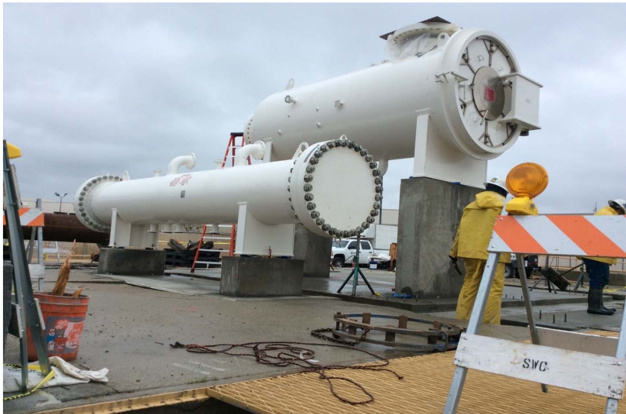
Figure 8: New Filter Separator Vessels
