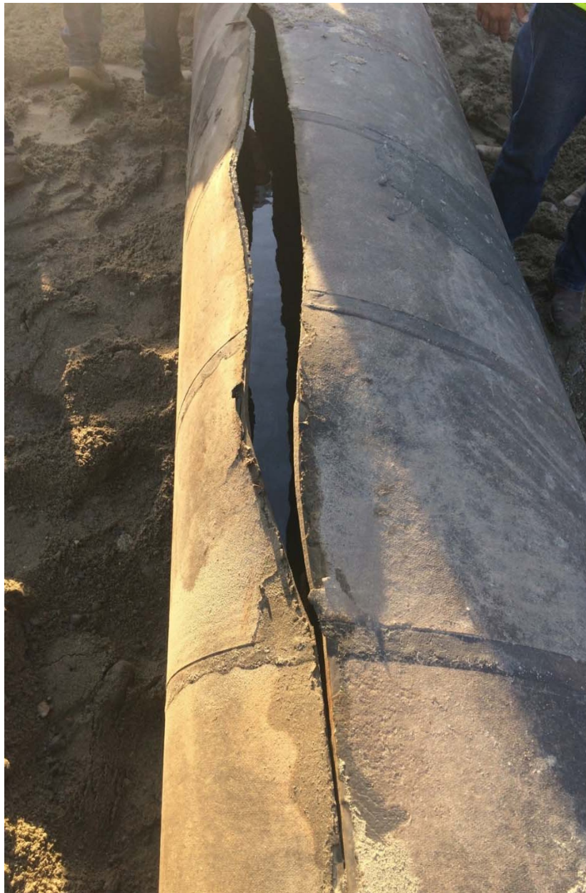
Figure 12: Hydrotest Rupture (close up)
