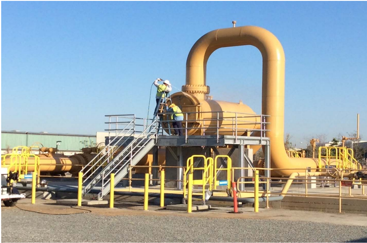
Figure 9: New Filter Separator
