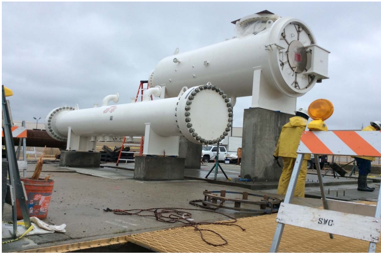
Figure 8: New Filter Separator Vessels
