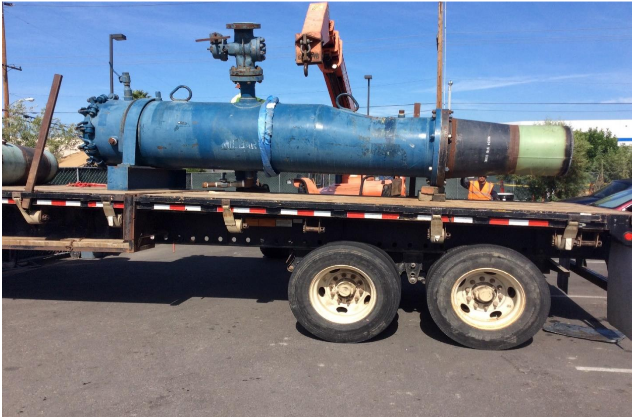
Figure 7: Off-loading Pig Launcher (used for launching multiple pigs for post hydrotest line drying)
