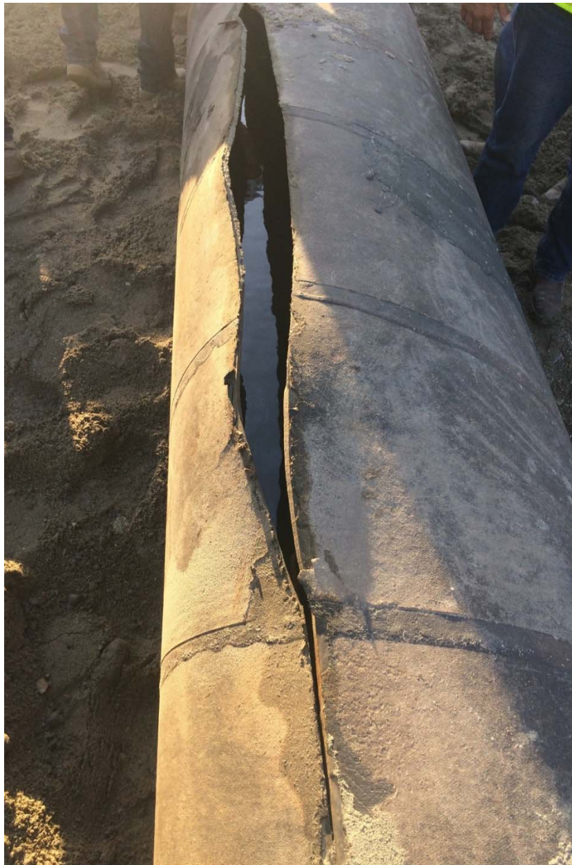
Figure 12: Hydrotest Rupture (close up)
