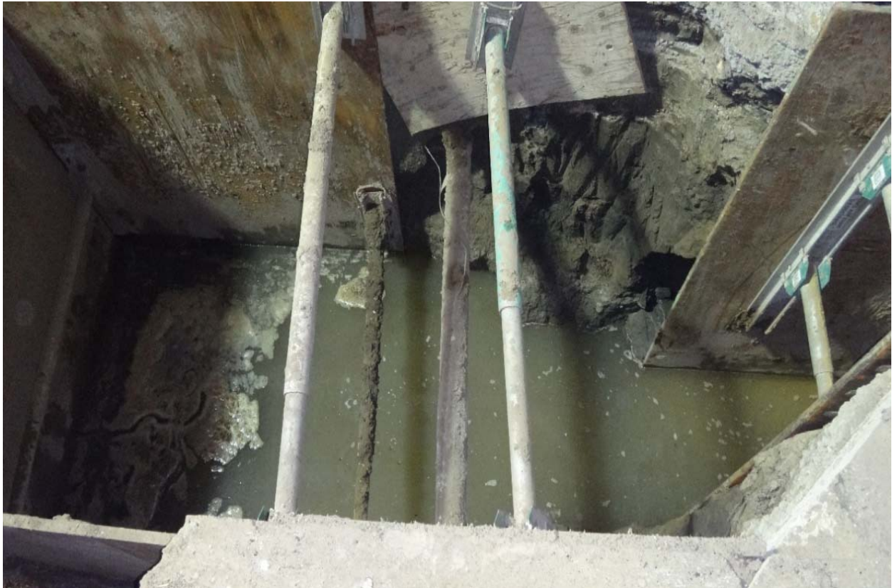
Figure 9: Groundwater Encountered During Excavation
