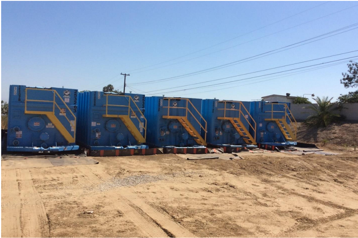
Figure 4: Water Storage Tanks for Hydrotest
