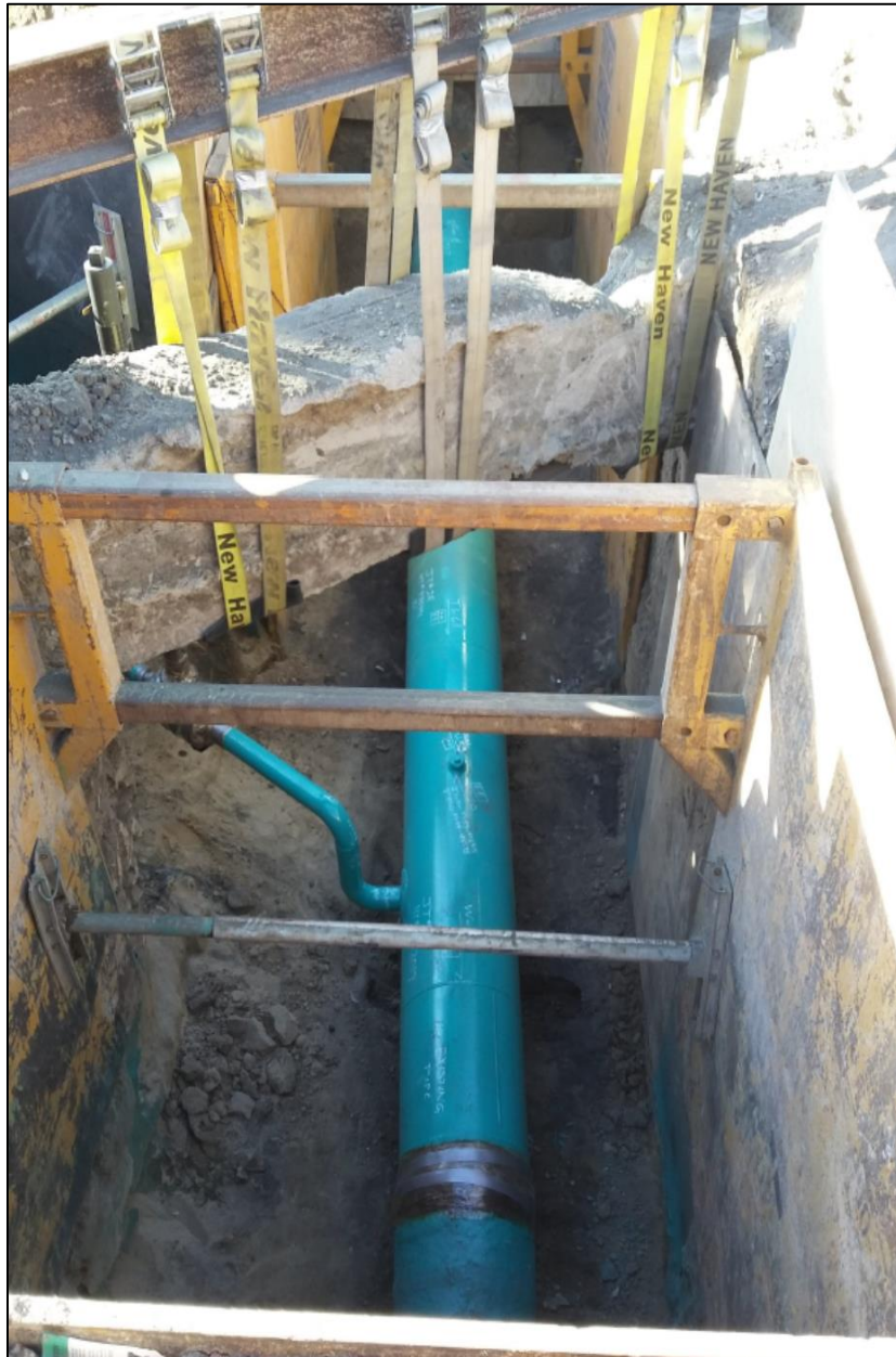
Figure 4: Tied-In Supply Line 31-09-H Lateral at Supply Line 31-09 South Hydrotest Test End
