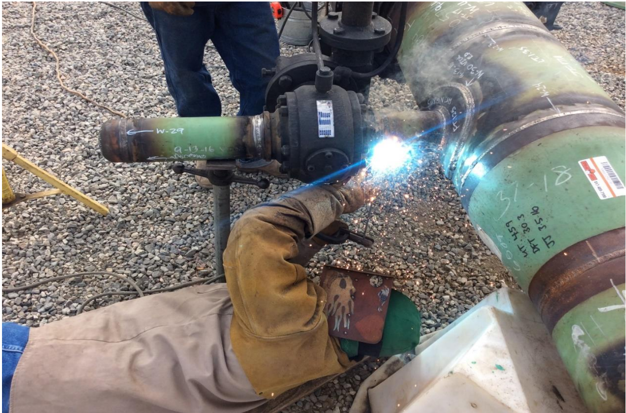
Figure 7: Fabrication of Bridle Tap and Valve on East Tie in Spool Added to Design
