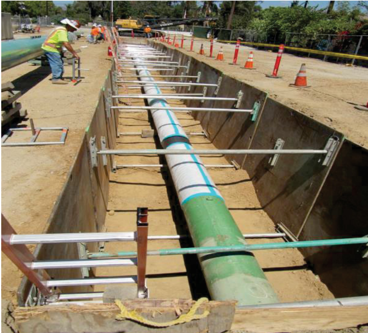
Figure 13: Exposed pipe on Section 5 with protective wrap in preparation for removal and asbestos abatement
