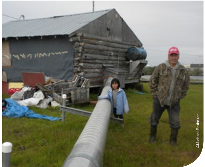
Rising temperatures are causing damage in Native villages in Alaska as sea ice declines and permafrost thaws. Resident of Selawik, Alaska, and his granddaughter survey a water line sinking into the thawing permafrost, August 2011.
