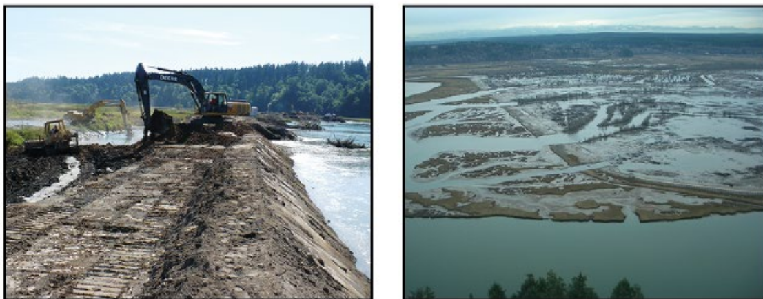
Figure 21.5. In Washington's Nisqually River Delta, estuary restoration on a large scale to assist salmon and wildlife recovery provides an example of adaptation to climate change and sea level rise. After a century of isolation behind dikes (left), much of the Nisqually National Wildlife Refuge was reconnected with tidal flow in 2009 by removal of a major dike and restoration of 762 acres (right), with the assistance of Ducks Unlimited and the Nisqually Indian Tribe. This reconnected more than 21 miles of historical tidal channels and floodplains with Puget Sound. 85 A new exterior dike was constructed to protect freshwater wetland habitat for migratory birds from tidal inundation and future sea level rise. Combined with expansion of the authorized Refuge boundary, ongoing acquisition efforts to expand the Refuge will enhance the ability to provide diverse estuary and freshwater habitats despite rising sea level, increasing river floods, and loss of estuarine habitat elsewhere in Puget Sound. This project is considered a major step in increasing estuary habitat and recovering the greater Puget Sound estuary. (Photo credits: (left) Jesse Barham, U.S. Fish and Wildlife Service; (right) Jean Takekawa, U.S. Fish and Wildlife Service).
