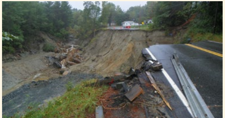
Figure 5.6. Vermont Route 131, outside Cavendish, a week after Tropical Storm Irene unleashed severe precipitation and flooding that damaged many Vermont roads, bridges, and rail lines. (Photo credit: Vermont Agency of Transportation).
