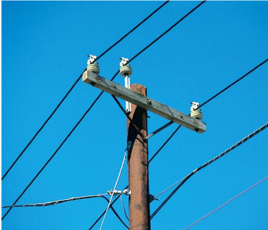
Figure 2. An example of crossarm-mounted CC, or “tree wire,” construction. Photo from Hendrix Aerial Cable Systems [Trager].
