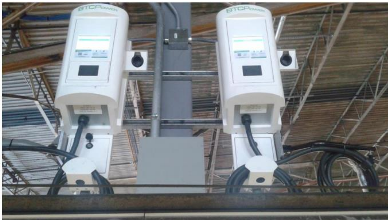
Figure 28. Fleet Delivery Equipment Installation
