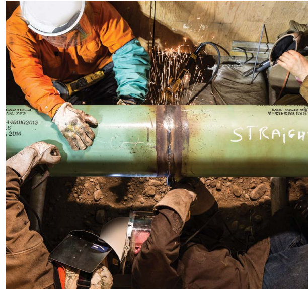
SDG&E has upgraded more than 36 miles of transmission pipeline in San Diego County as part of our Pipeline Safety Enhancement Plan.
