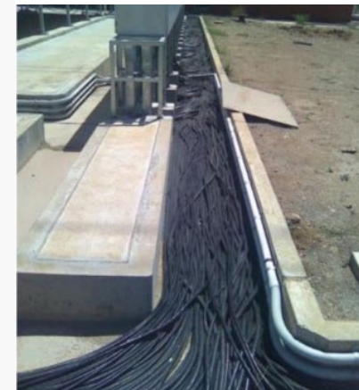
Hard wired substation
