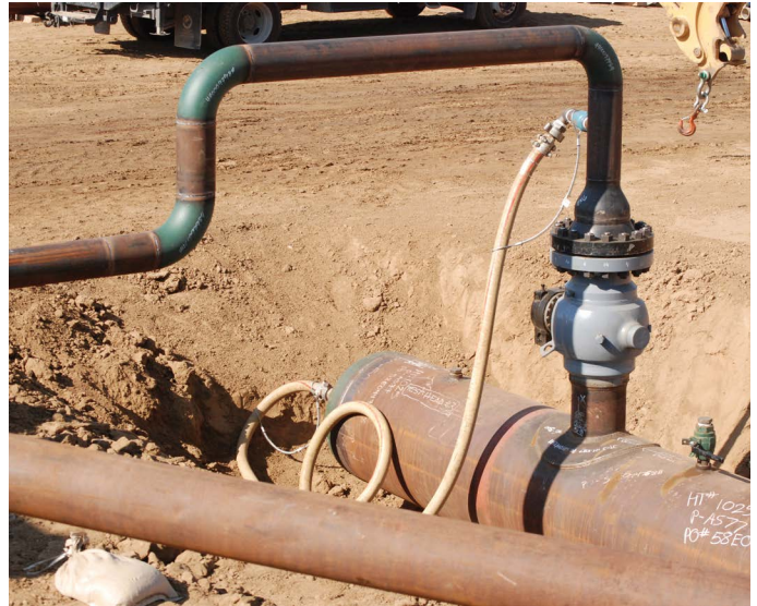
Water is pumped into a test head to conduct a strength test.
