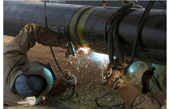
A pipeline test head cap is carefully welded to the end of a pipeline segment to be strength tested.
