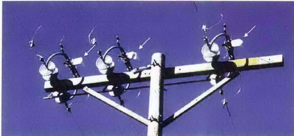
Figure 3-14 600 Amp KPF Air Switch, Crossarm Construction (closed position) With Arcing Horns and Snuffers
