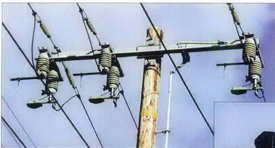
Figure 3-16 600 Amp Underarm Sidebreak Switch (open position)
