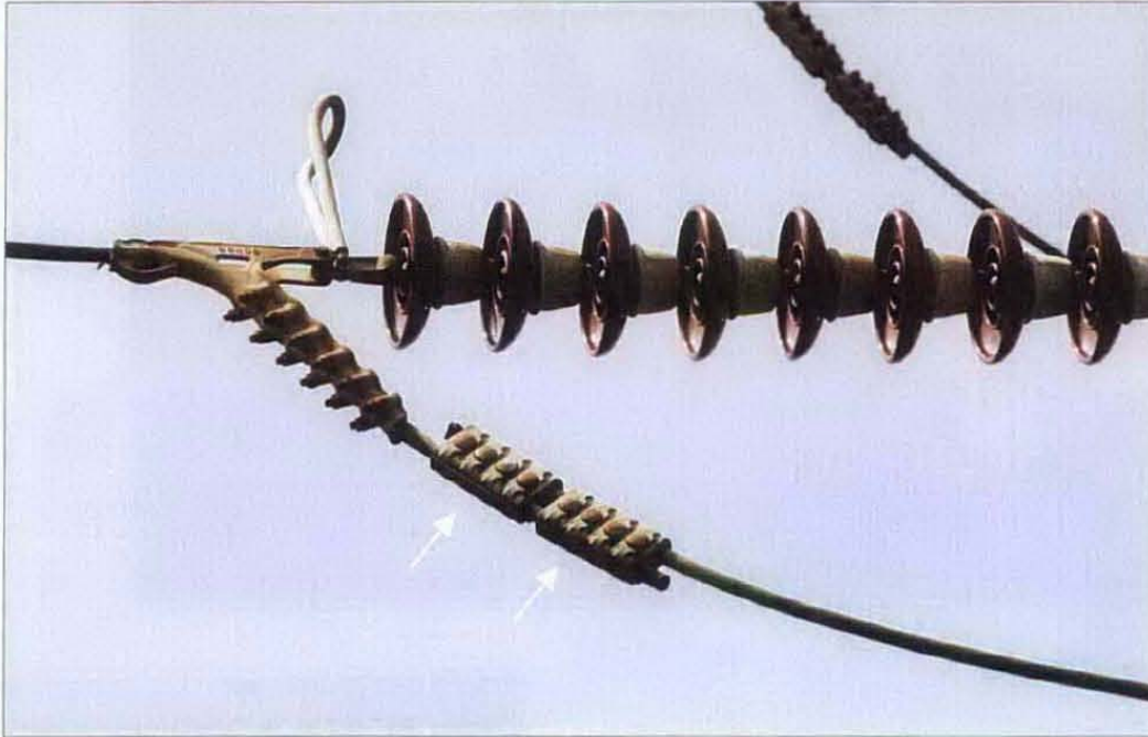
Figure 3-34 Transmission Deadend with Parallel Groove Connectors
