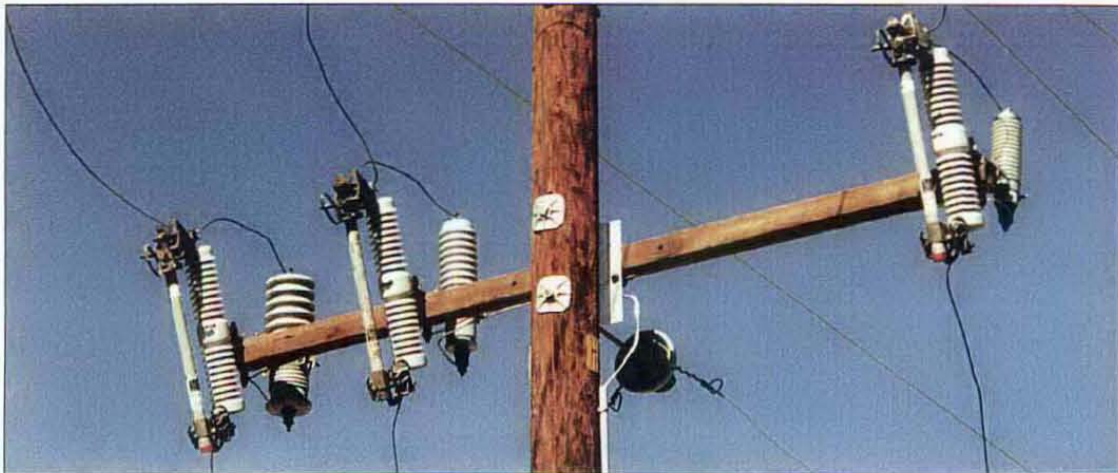
Figure 3-10 Arm Mounted Cutout with SMU-20 Fuses
