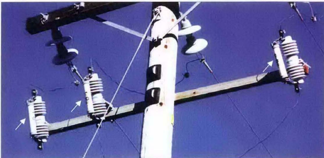
Figure 3-3 Arm Mounted Cutout with Non-Expulsion Fuses
