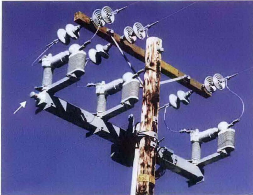
Figure 3-22 S&C Scada-Mate Switch
