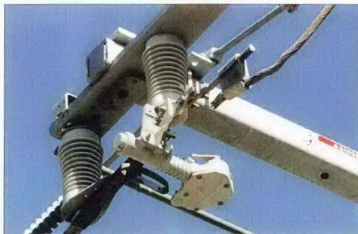
Figure 3-19 S&C Underarm Side-Break Switch (closed position)
