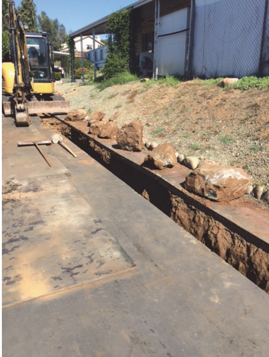
Fig. 5: Hard-digging leads to unforeseen costs that cannot be predicted during design. In this instance, it took several days to break through blue granite at Heart O' the Hills. Discovery of boulders in the trench route can also increase dump fees.
