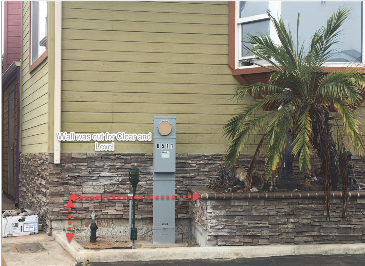
Fig.13: Maintaining a clear and level workspace around the gas and electric metering facilities per SDG&E standards sometimes requires modifications to the current mobile home layout
