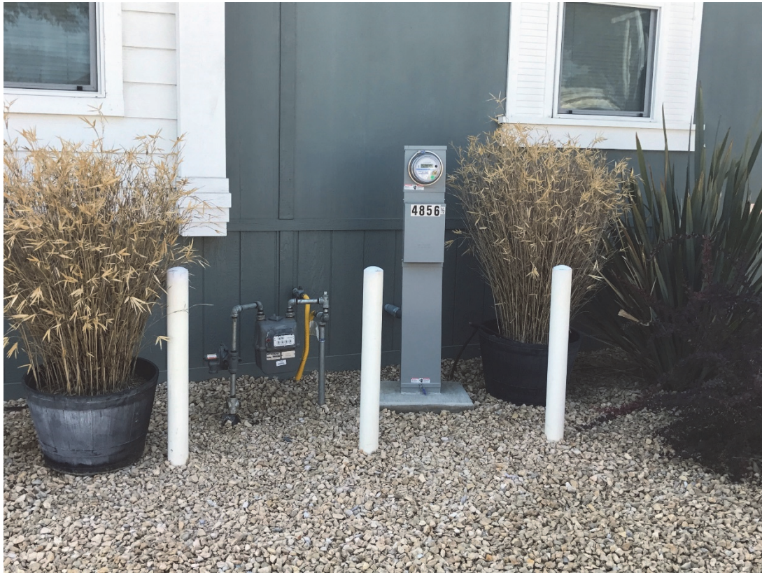
Fig. 15: Newly installed gas and electric meters and protective bollards at the front of a mobile home lot
