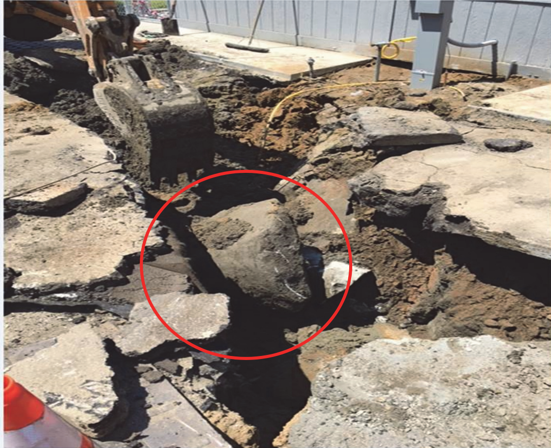
Fig. 6: Hard-digging leads to additional costs that cannot be predicted during design and estimation. In this instance at Westward Ho, it took several days to break through rock, causing unforeseen dumping fees and unavoidable pavement repairs.
