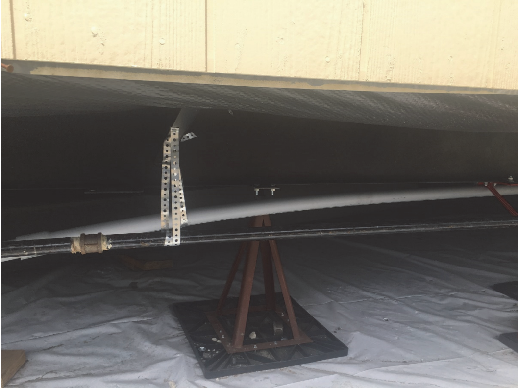
Fig. 11: Gas and electric house lines on hangers per HCD inspection and installation guidelines
