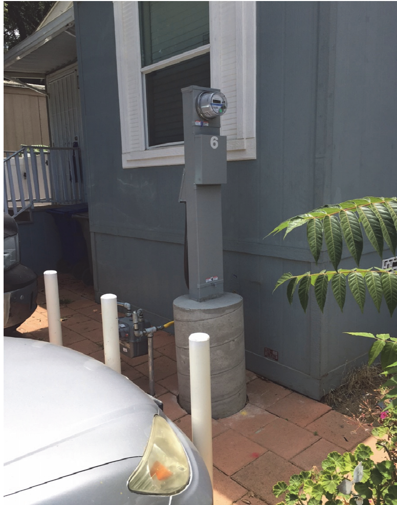
Fig.14: Unexpected changes can occur in the scope of work. In this instance, due to FEMA flood zone requirements, the BTM Contractor had to install a concrete pier for the pedestal to raise it to sufficient height.
