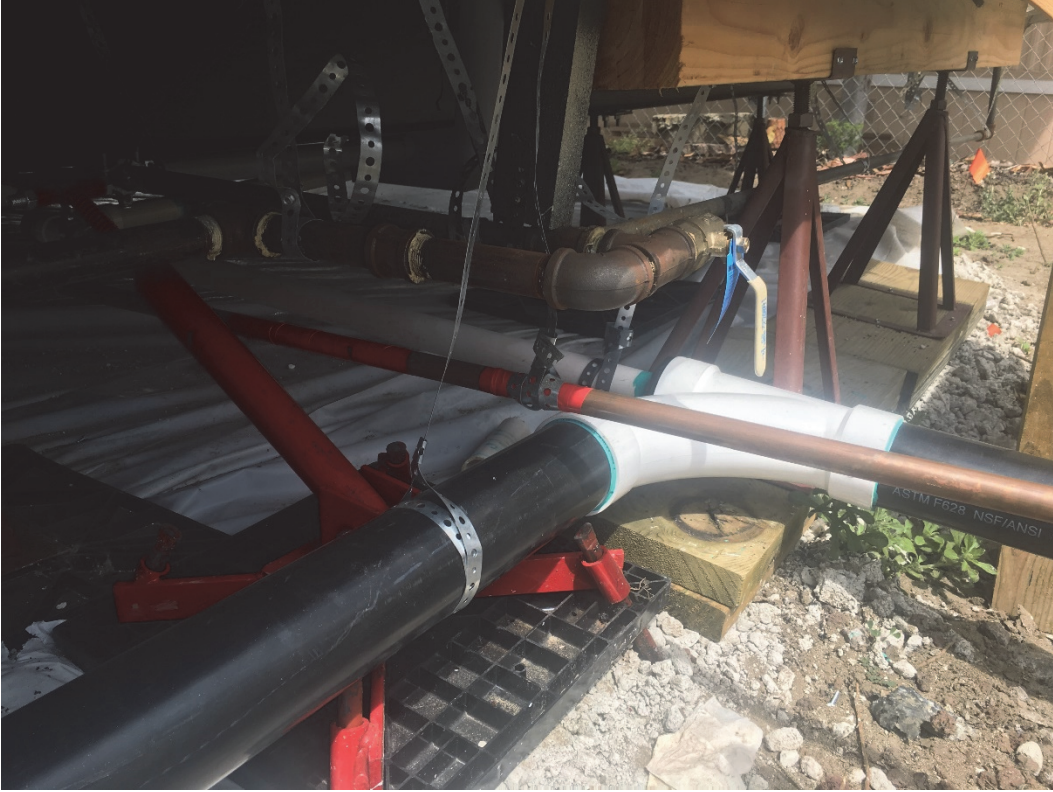
Fig. 12: Gas and electric house lines on hangers per HCD inspection and installation guidelines
