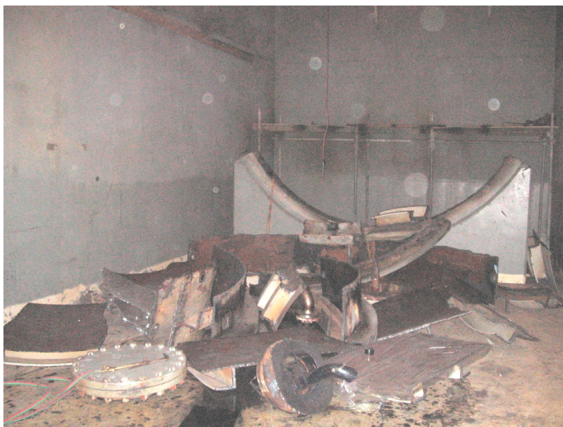
Figure III-18 Debris from Hold Up Tank in Lower Radwaste Building
