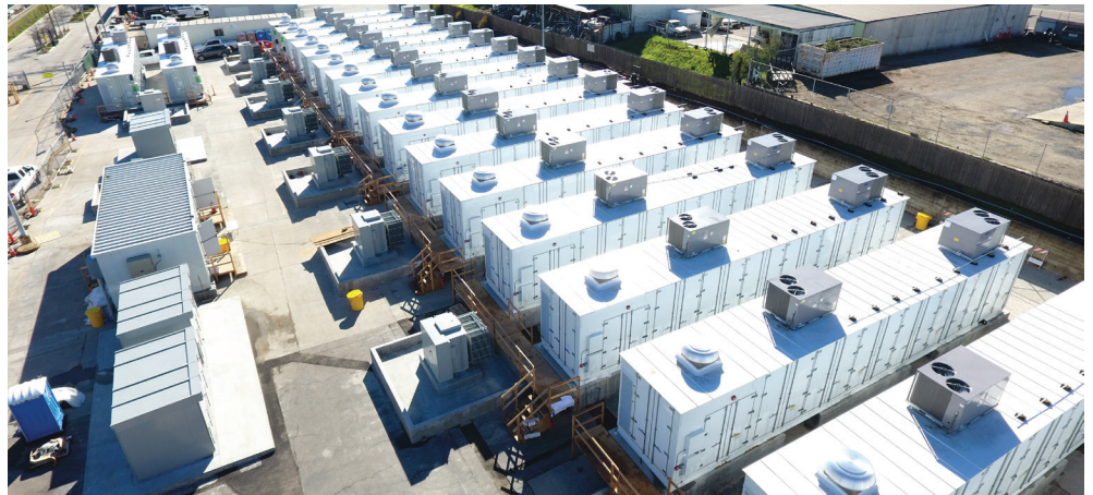
Escondido Battery Energy Storage System project
