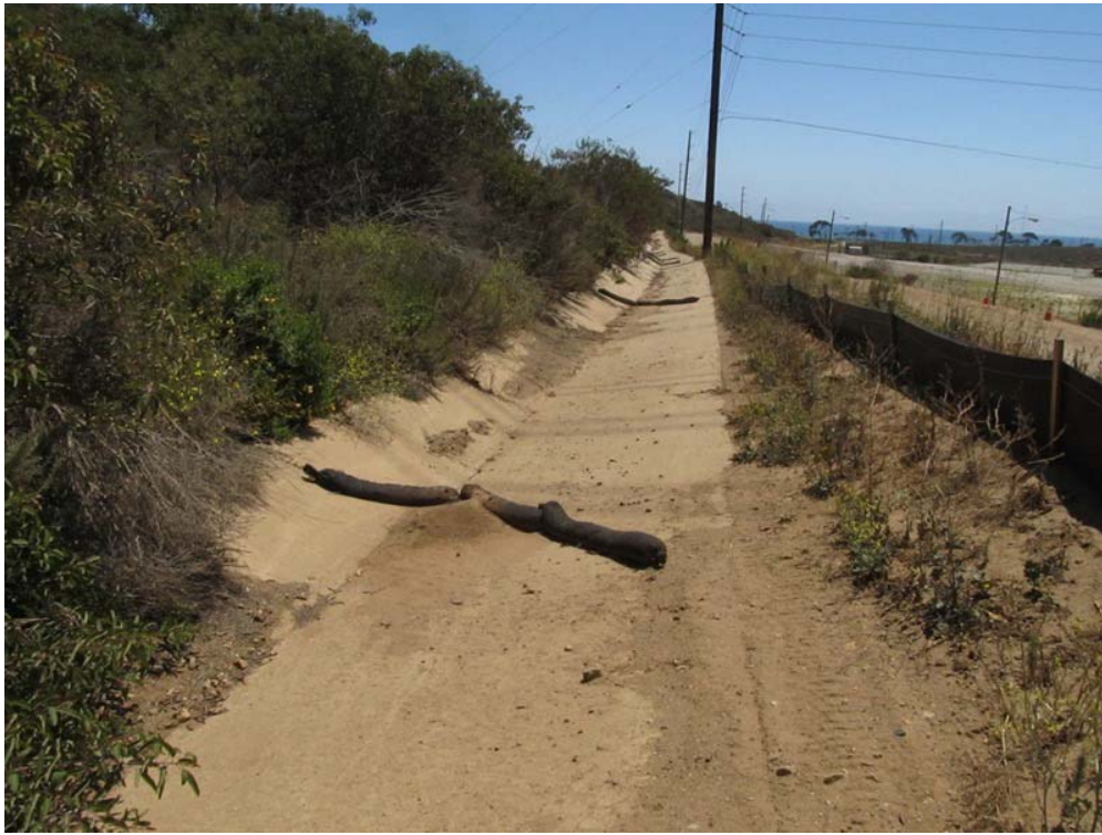
Photograph 35 (Southwest of SONGS Mesa Facility, Mapbook Pages 32 and 33): Non-jurisdictional concrete brow ditch south of the SONGS Mesa Facility. View west.
