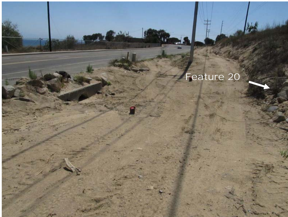
Photograph 44 (West of Pole 76, Mapbook Page 37): Feature 20 end, graded area between feature and culvert inlet. View west.
