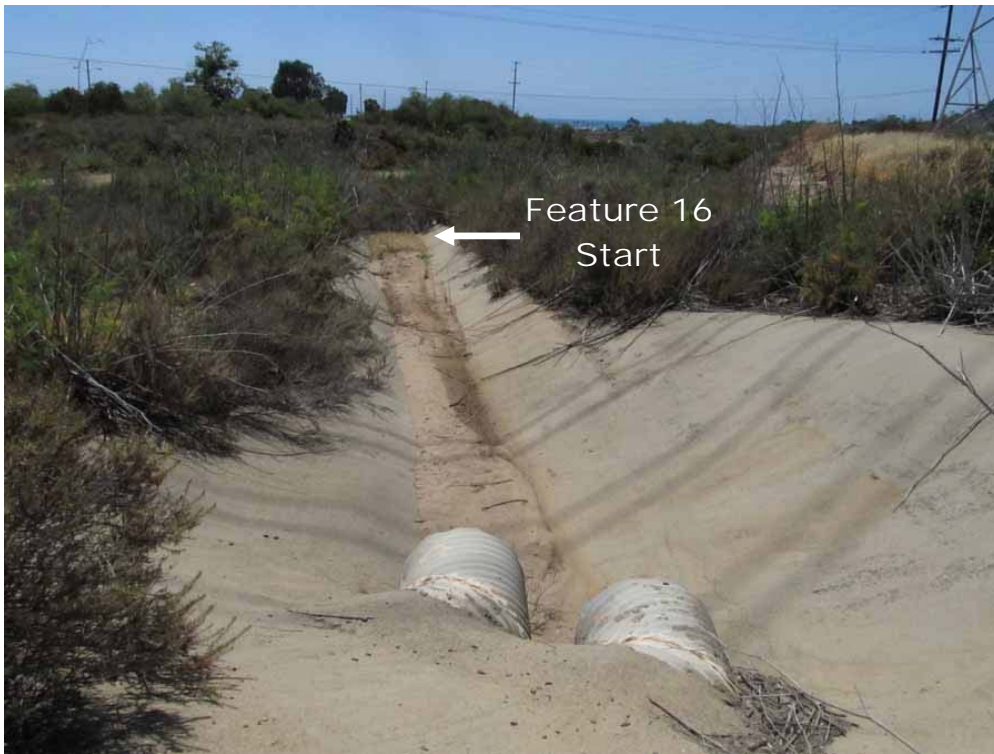
Photograph 31 (Between Poles 88 and 56, Mapbook Page 30): Feature 16, ephemeral channel at the end of concrete ditch. View west.
