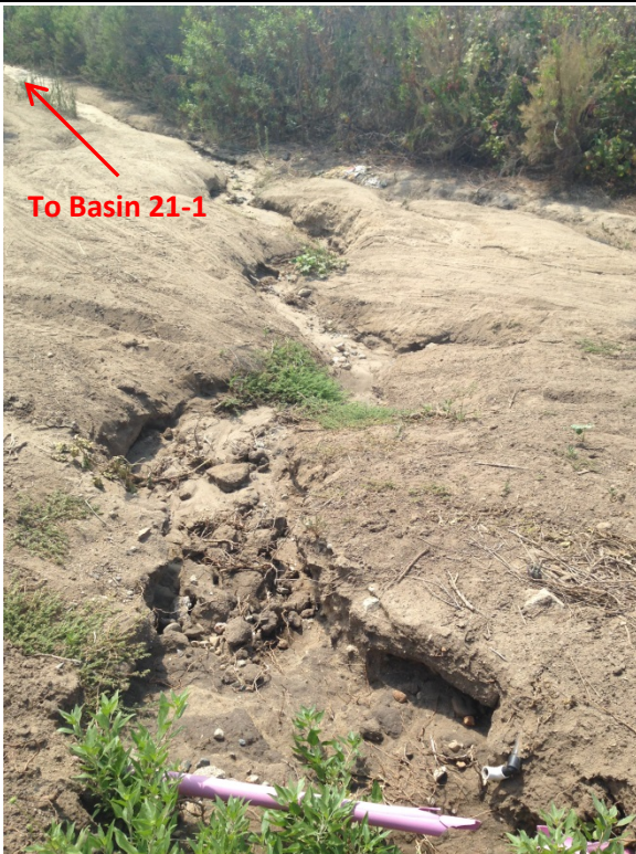
View downslope from burst pipe. Photo by RCS, 9 Sep 2015.
