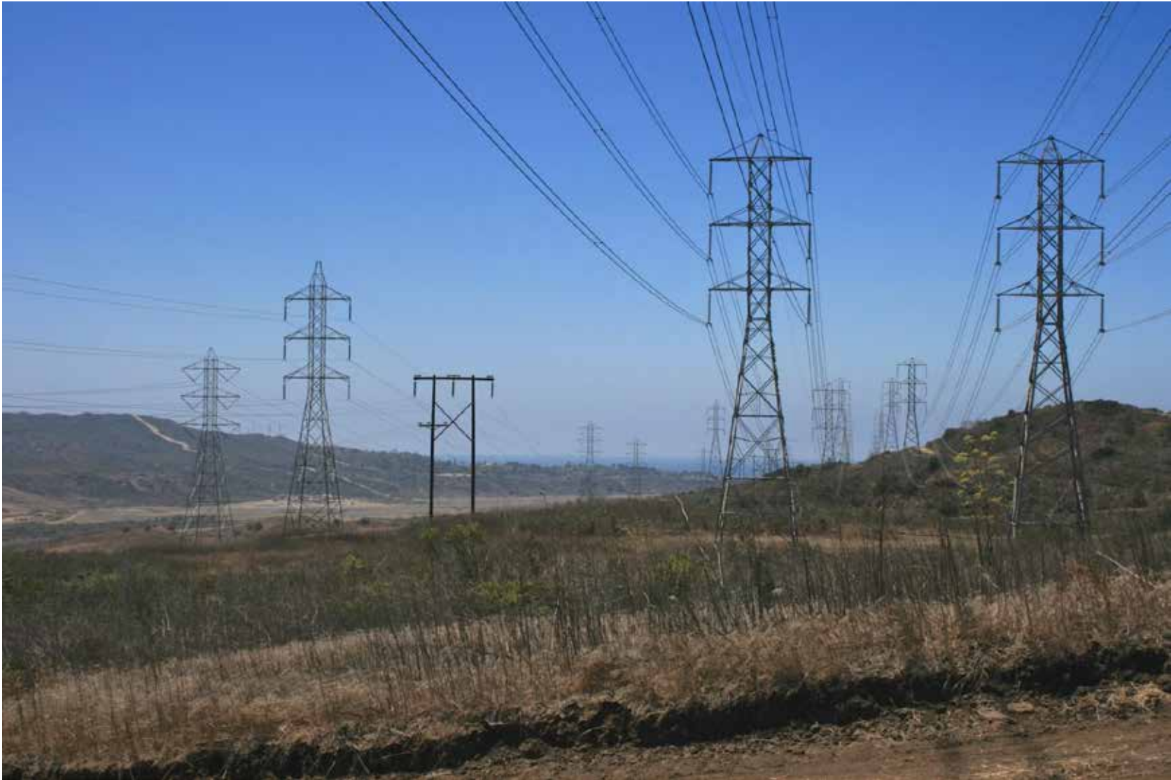
Key Observation Point#13: Existing view looking south from SDG&E access road at power line H-frame structure See Figure 4.1-1 for viewpoint location
