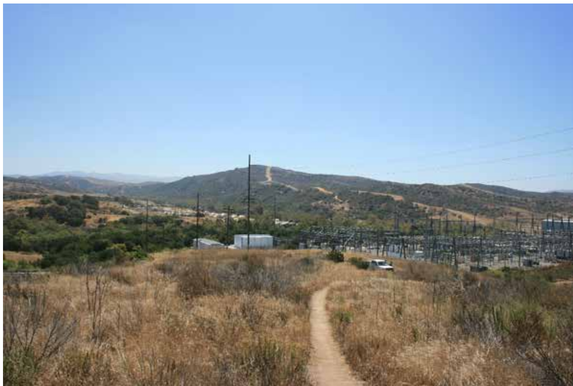
Viewpoint 6: Existing view looking southeast from SDG&E access road at Talega Substation.
