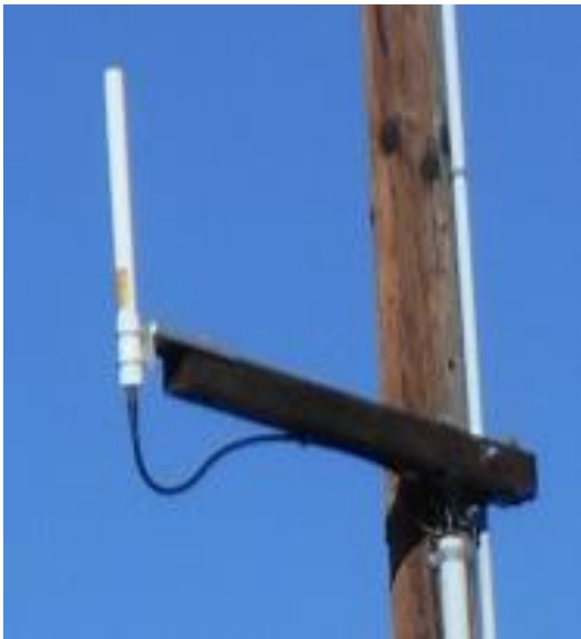
Single crossarm, no bracing, supporting incidental wiring and omni-directional rod
