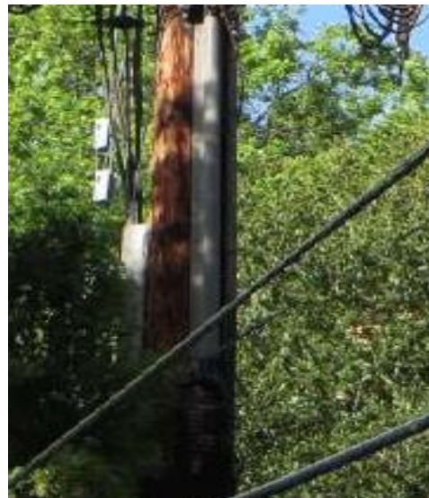
Vertical Cable Risers (Covered and Uncovered)
