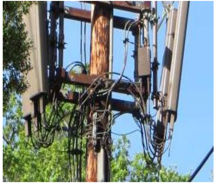
Two sets of double crossarms, w/o bracing, supporting wires, pipe brackets and directional panels
