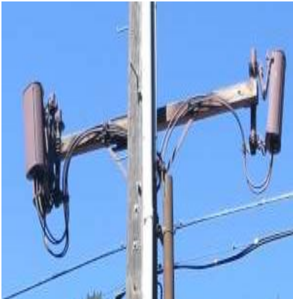
Single crossarm, w/bracing supporting incidental wiring, and pipe brackets, w/directional panels
