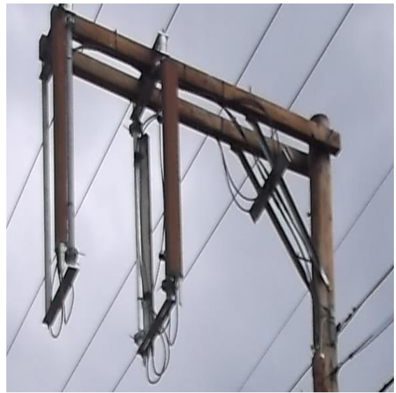
Double crossarms (alley arms) w/braces, supporting incidental wiring and pipe brackets w/directional panels
