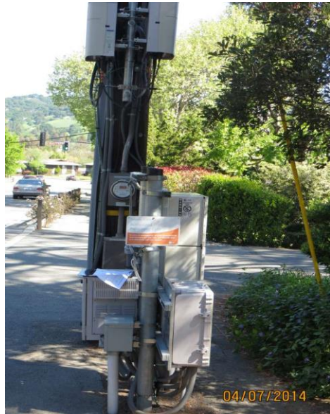
Cellular/PCS equipment (Ground and Pole Mounted)
