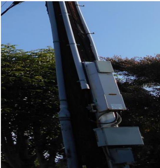
Vertical cable riser and Electric service vertical risers
