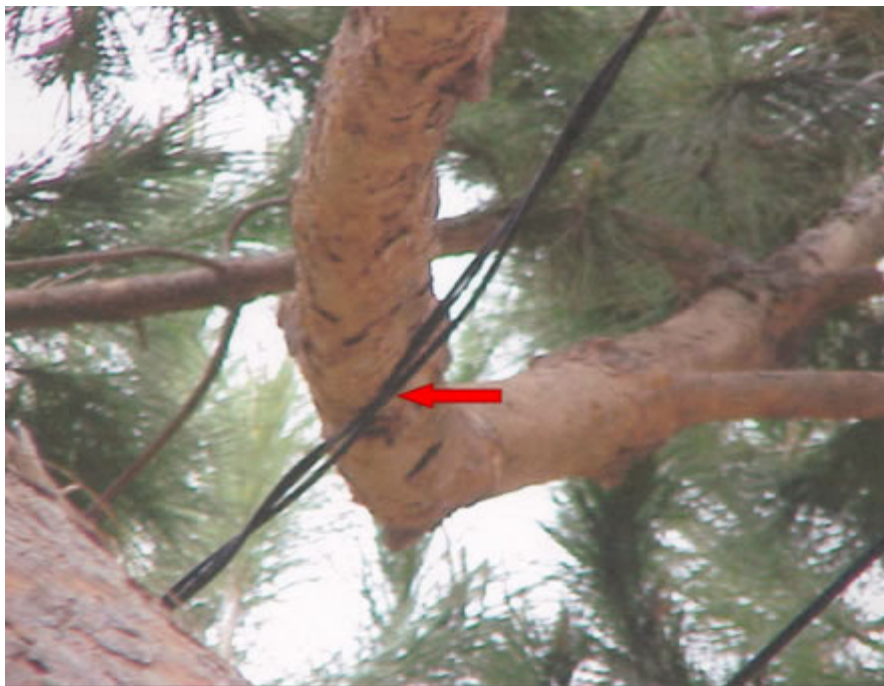
Reroute – Vegetation in Service Pole to House Code 325
