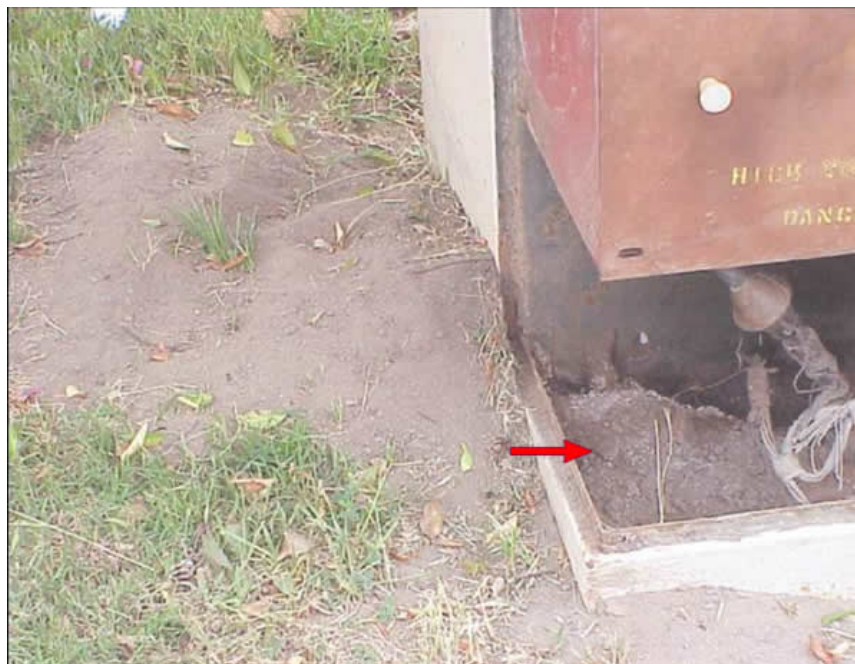
Weeds, Grass, Dirt Inside Unit (Clear On Site) Code 74
