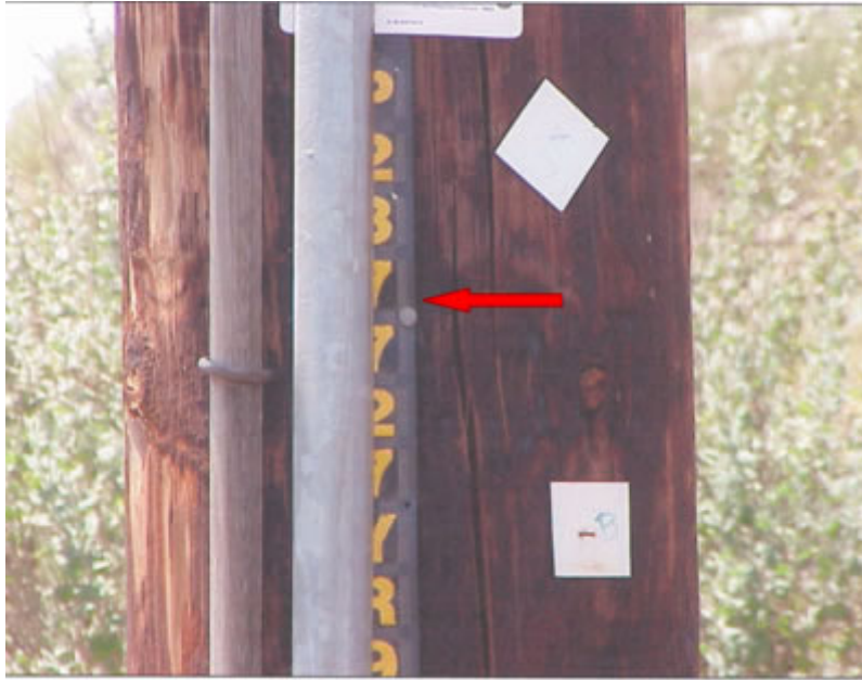
ID Missing, Damaged or Incorrect Code 283
