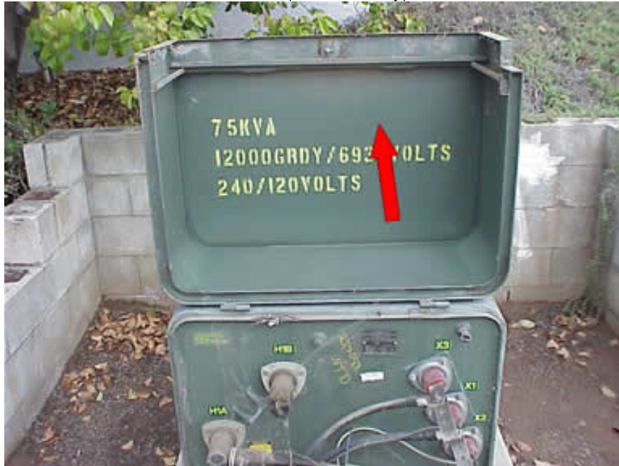
High Voltage Sign Damaged or Missing (Deadfront) Code 4 (Discretionary)
