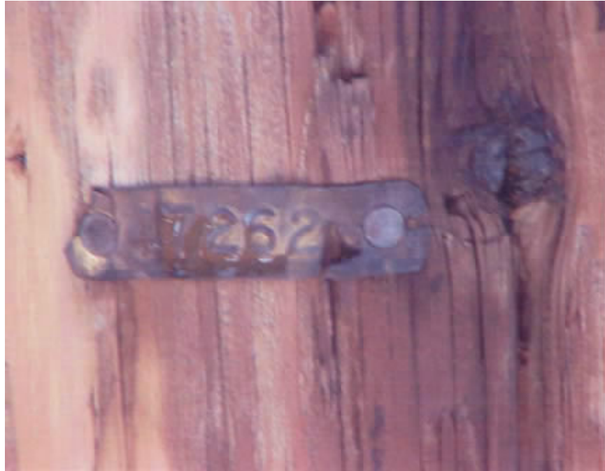
ID Missing, Damaged or Incorrect Code 283
