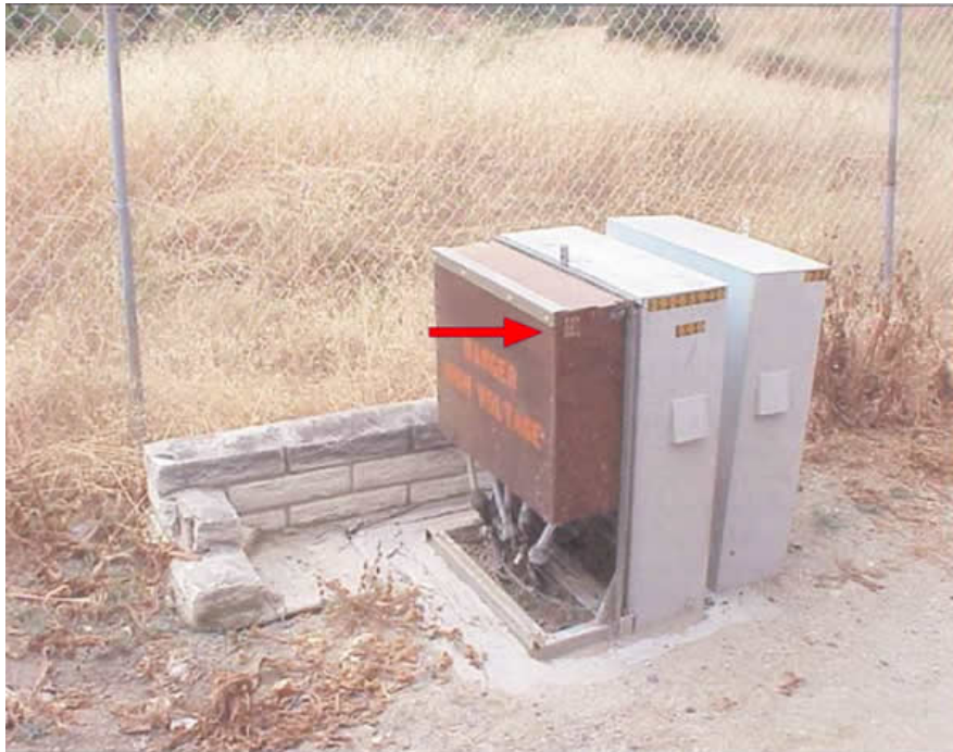
High Voltage Sign Damaged or Missing (Livefront) Code 5 (Infraction)
