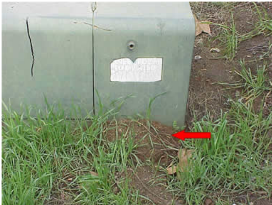
Weeds, Trees, Bushes, Dirt or Obstacle Outside Unit Code 47
