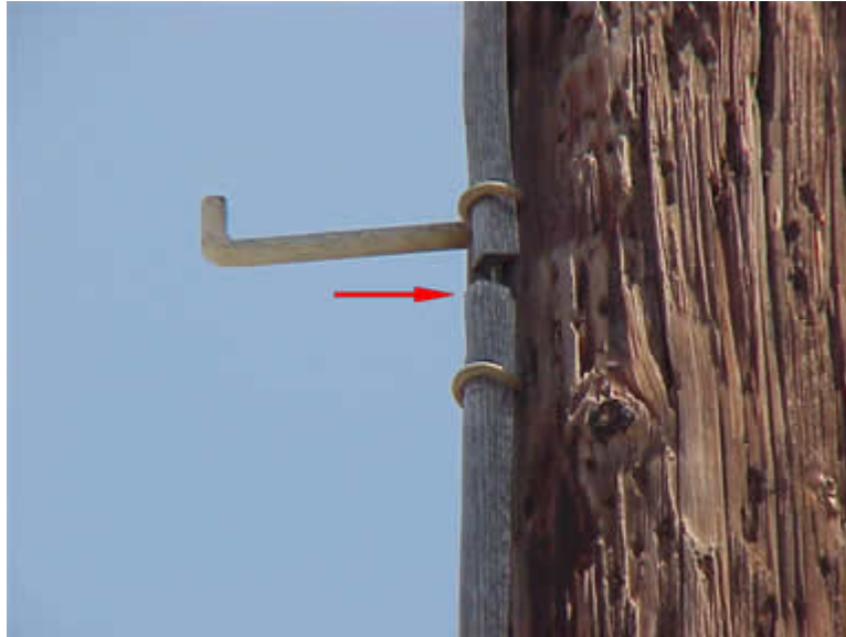
Damaged Ground Molding Code 230
