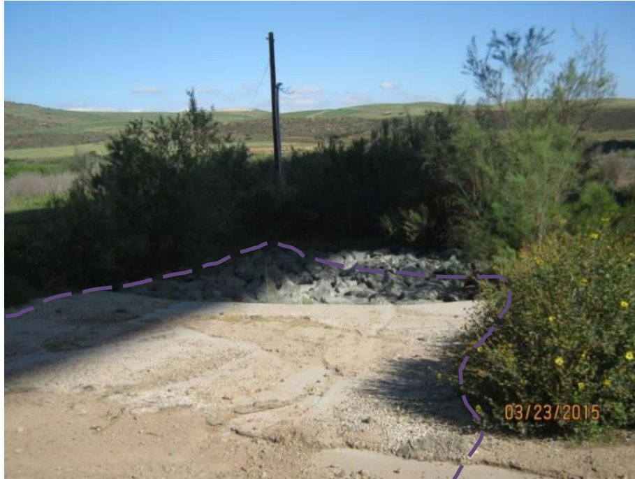
Photograph 17: Feature 17 is a non-jurisdictional concrete brow ditch and energy dissipater east of Locations 50.1 and 50.2. Feature 17 sheet flows across a maintained, concrete Arizona crossing on an existing project access road. Photograph taken facing north.
