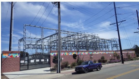
Otay Substation, looking southeast. March 23, 2015
