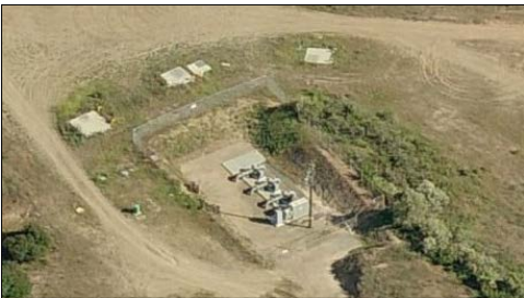
Otay Lake Substation (Pictometry.com 6/13/2006)
