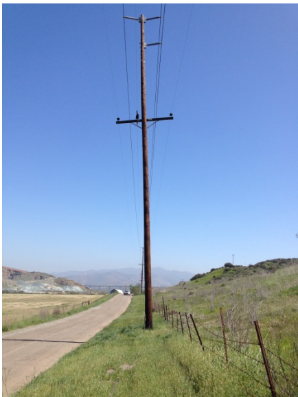
View of pole 188728.
