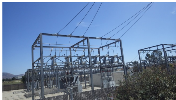
Border Substation, looking southeast. March 23, 2015
