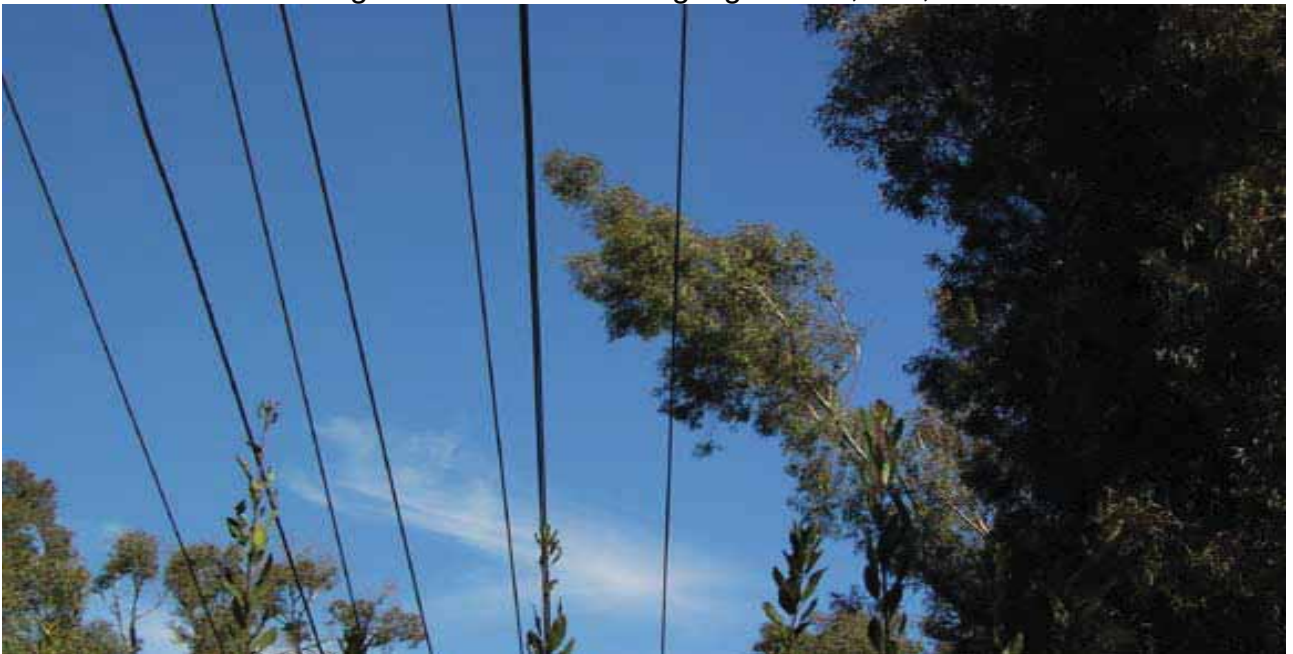
Figure 13: Minutes later the winds pick up and the tree may now pose a potentially hazard. Keep in mind pre-inspection must anticipate tree and weather conditions through all seasons including high winds, rain, and snow.
