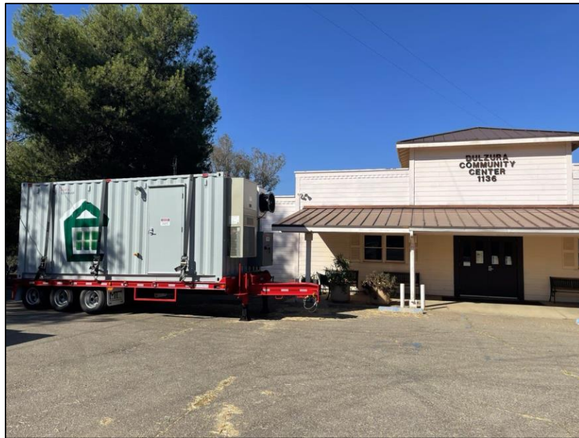
Figure 5-3. Picture of the MBESS in Front of the Dulzura CRC for Demonstration 1
