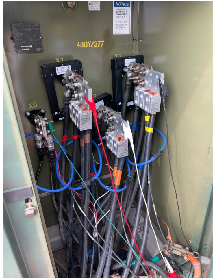
Figure 2: MBESS Connection to MGBW Transformer
