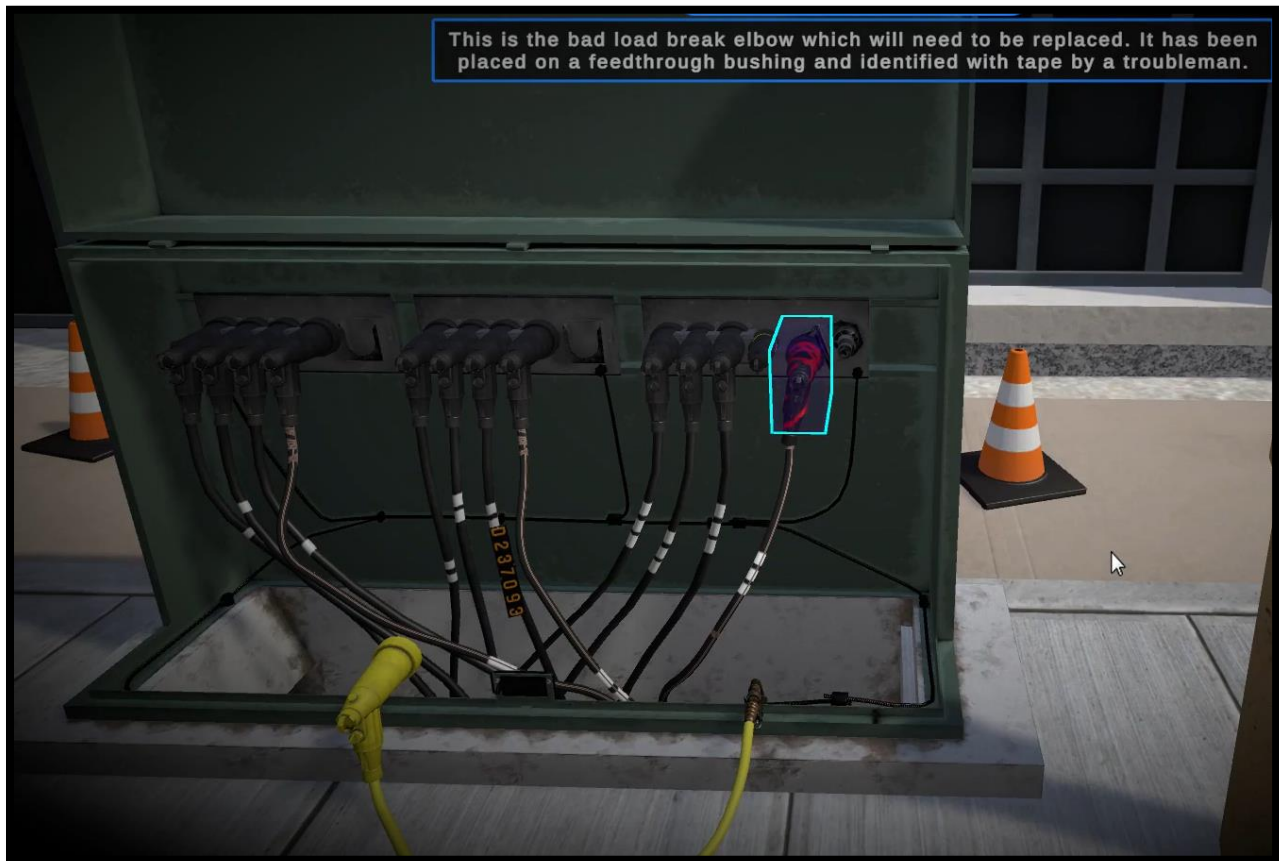
Figure 2: Faulty Load Break Elbow
