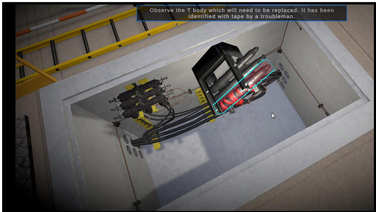
Figure 4: Failed 600-AMP T Connector
