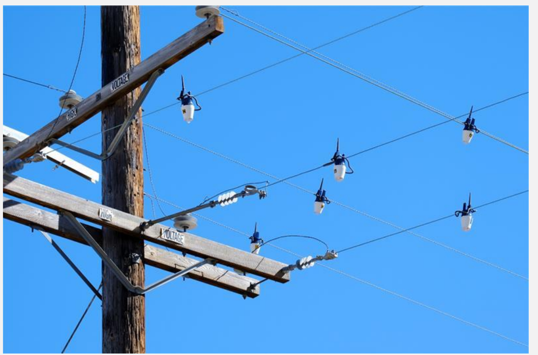
Fig. 2. Wireless Fault Indicator (WFI) Devices installed in the field
