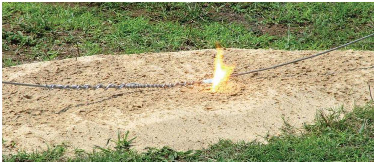
Figure 12.2: Energized Downed Conductor Causes Arcing – Potential Safety Hazard
