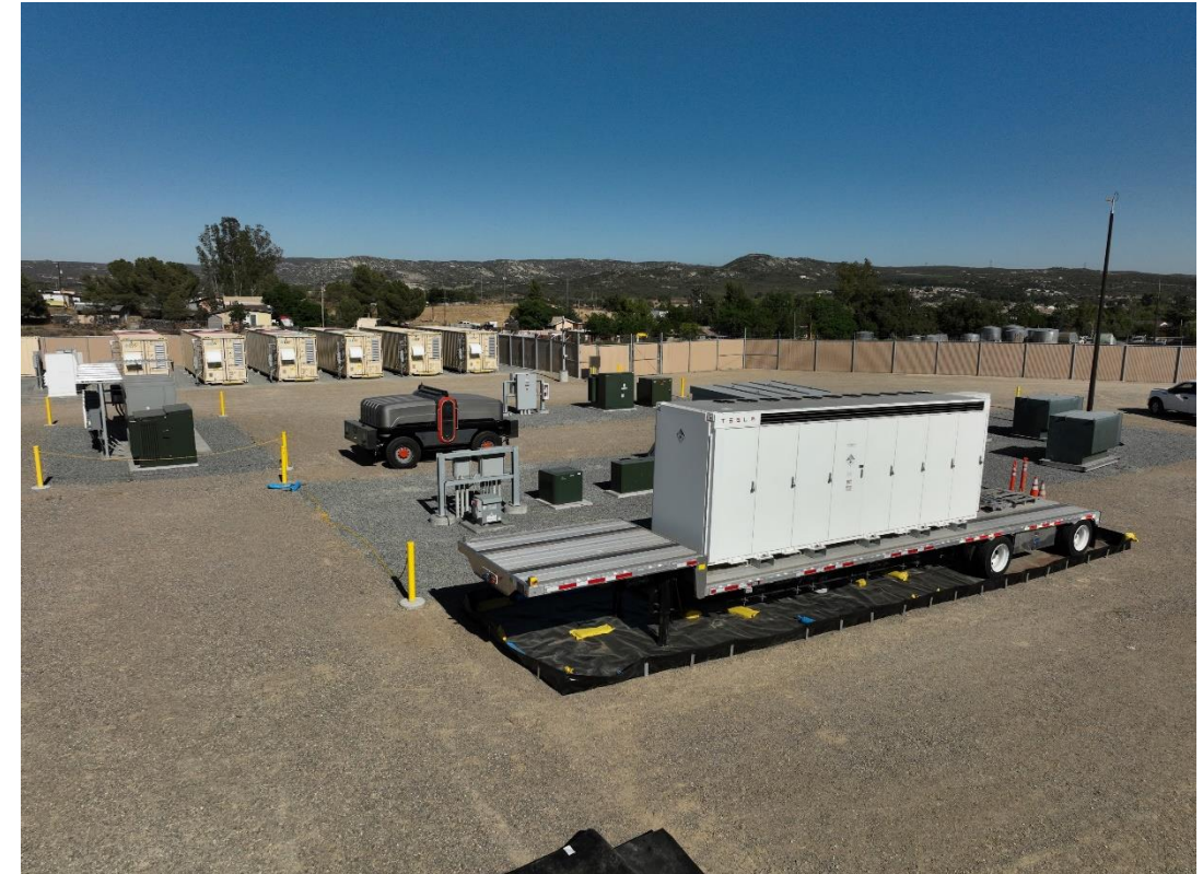
MBESS at Cameron Corners Microgrid
