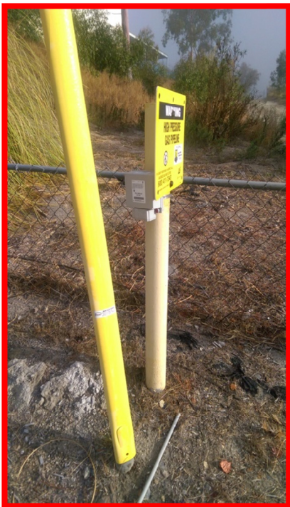
Figure 4 Methane sensor on ROW marker
