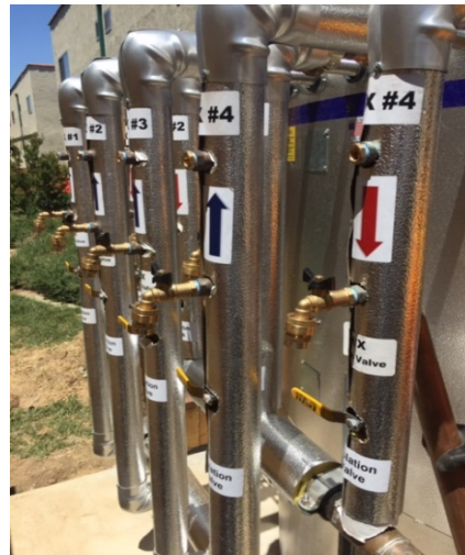
Solar thermal heat exchanger piping
