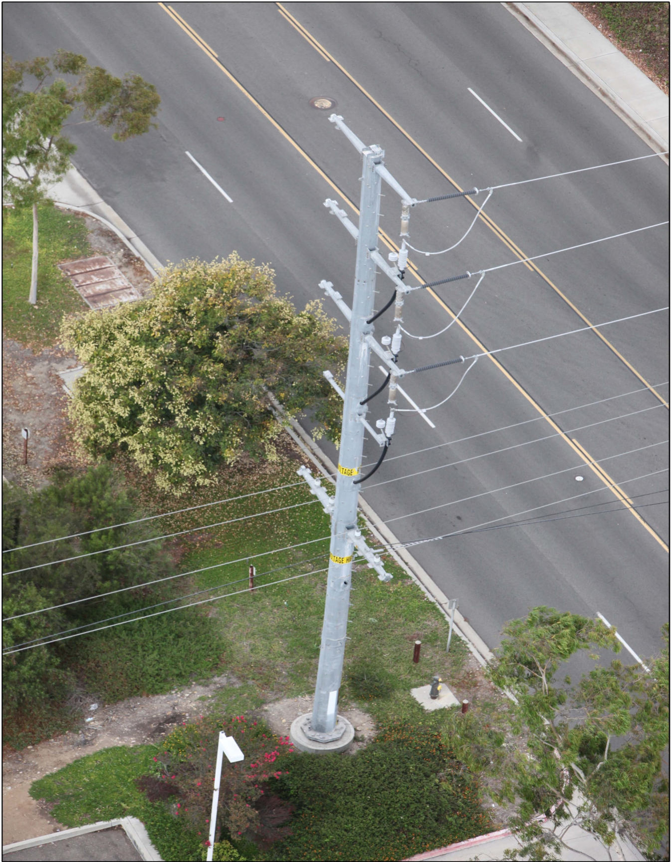
Typical 69kV Double-Circuit Cable Pole with Only 1 Side Installed & Distribution Underbuild
