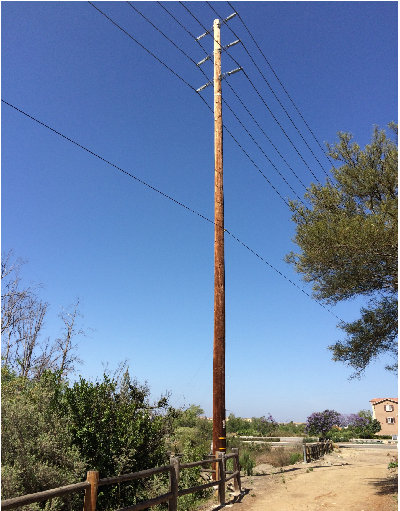
Typical 69kV Double-Circuit Tangent Wood Monopole
