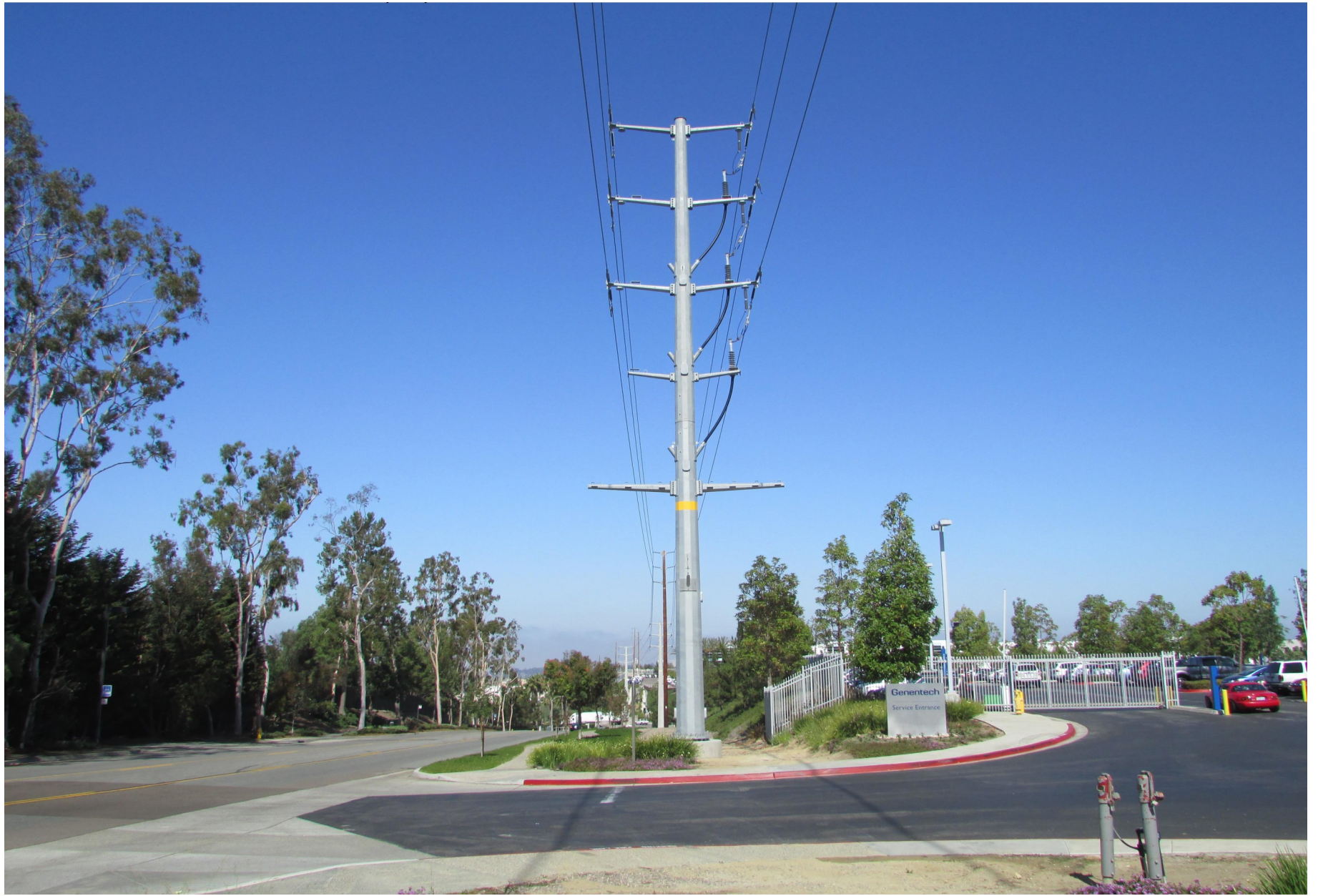
Typical 69kV Double-Circuit Steel Cable Pole with Only 1 Side Installed and 1 Side Pass Through
