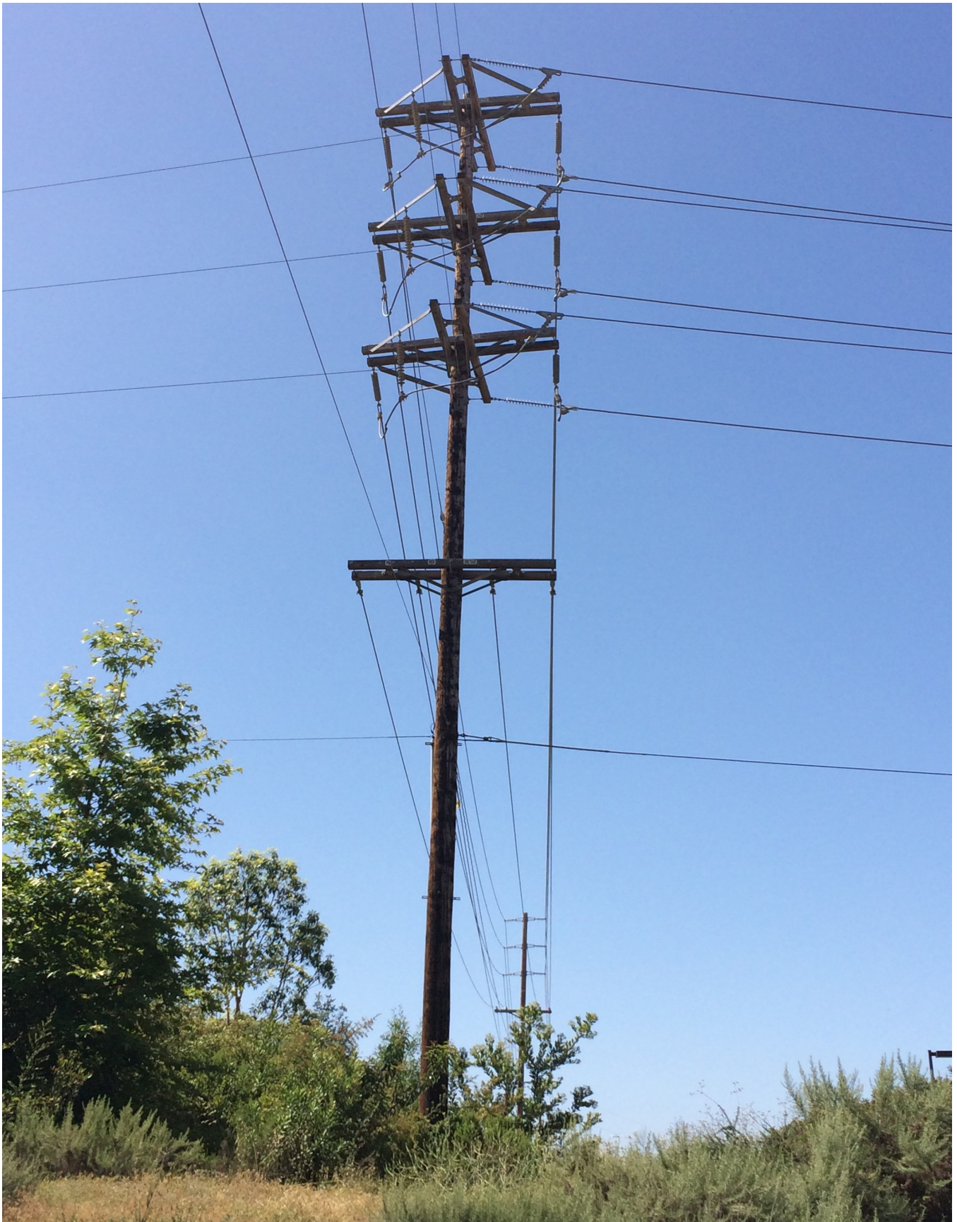
Typical 69kV Double-Circuit Dead-end Wood Monopole with Distribution Underbuild
