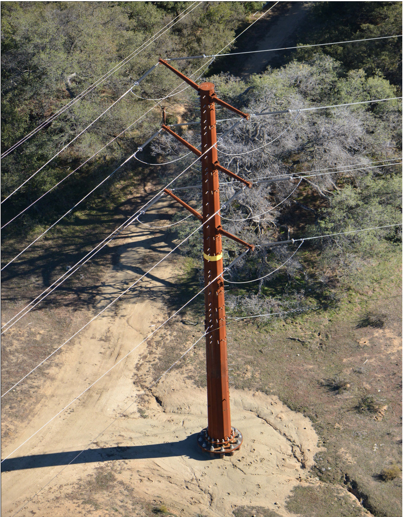
Typical 69kV Double-Circuit Dead-end Weathering Steel Tubular Pole
