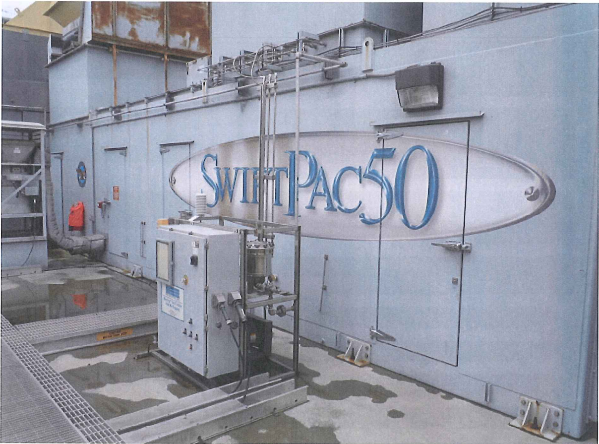
Gas Turbine Package
