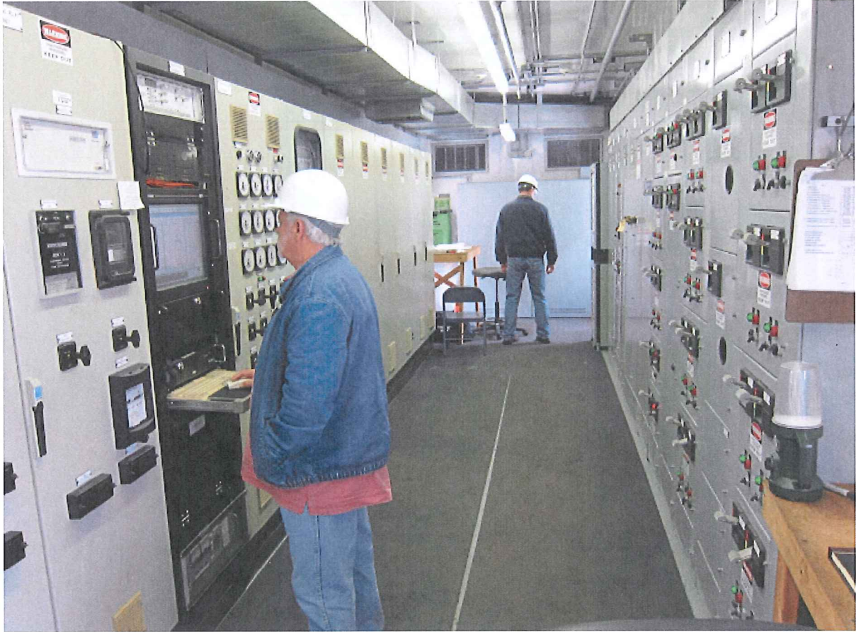
Electrical Package MCC and Control Center
