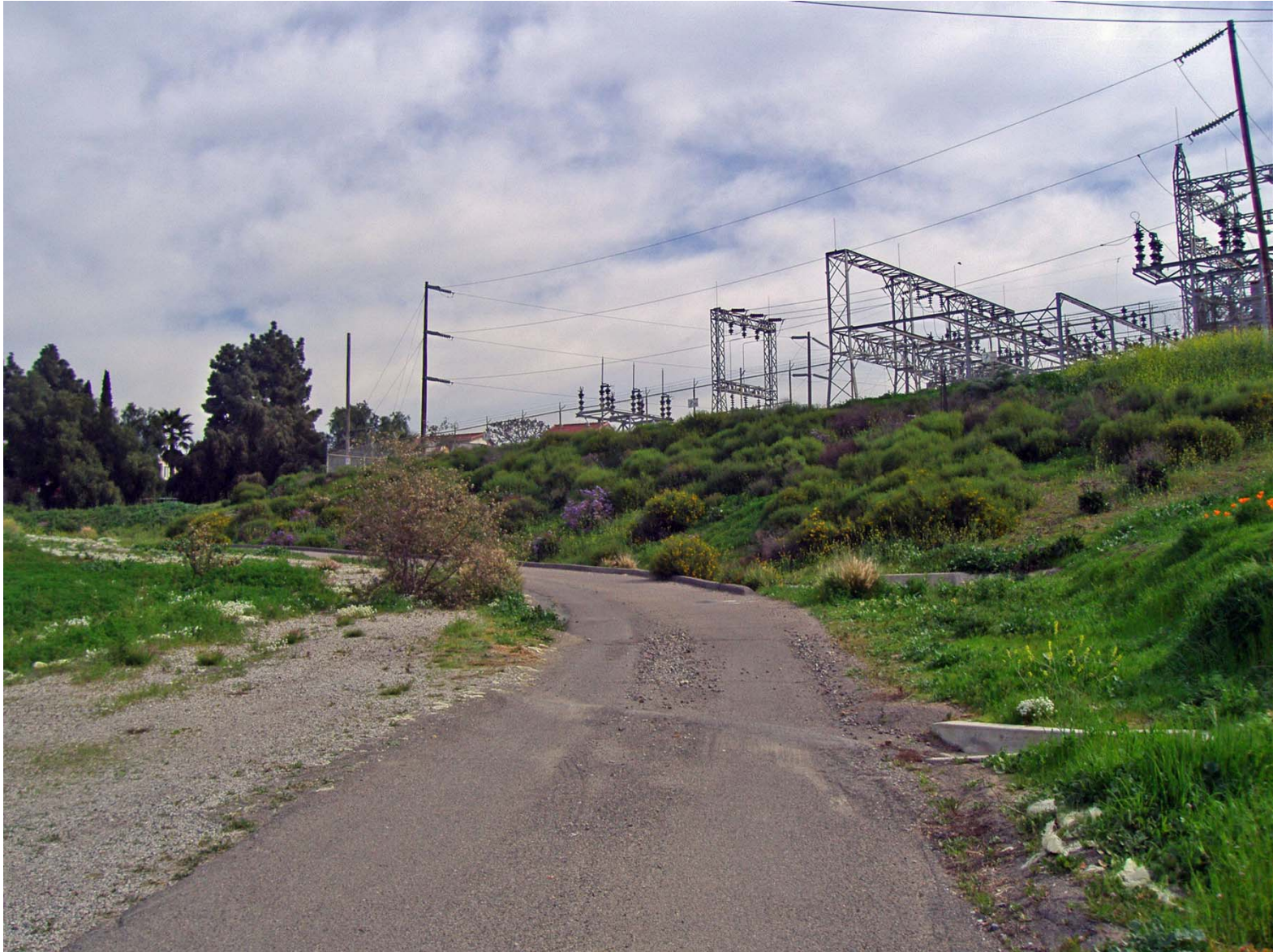
Asphalt road Leading to Modern Substation (facing East).
