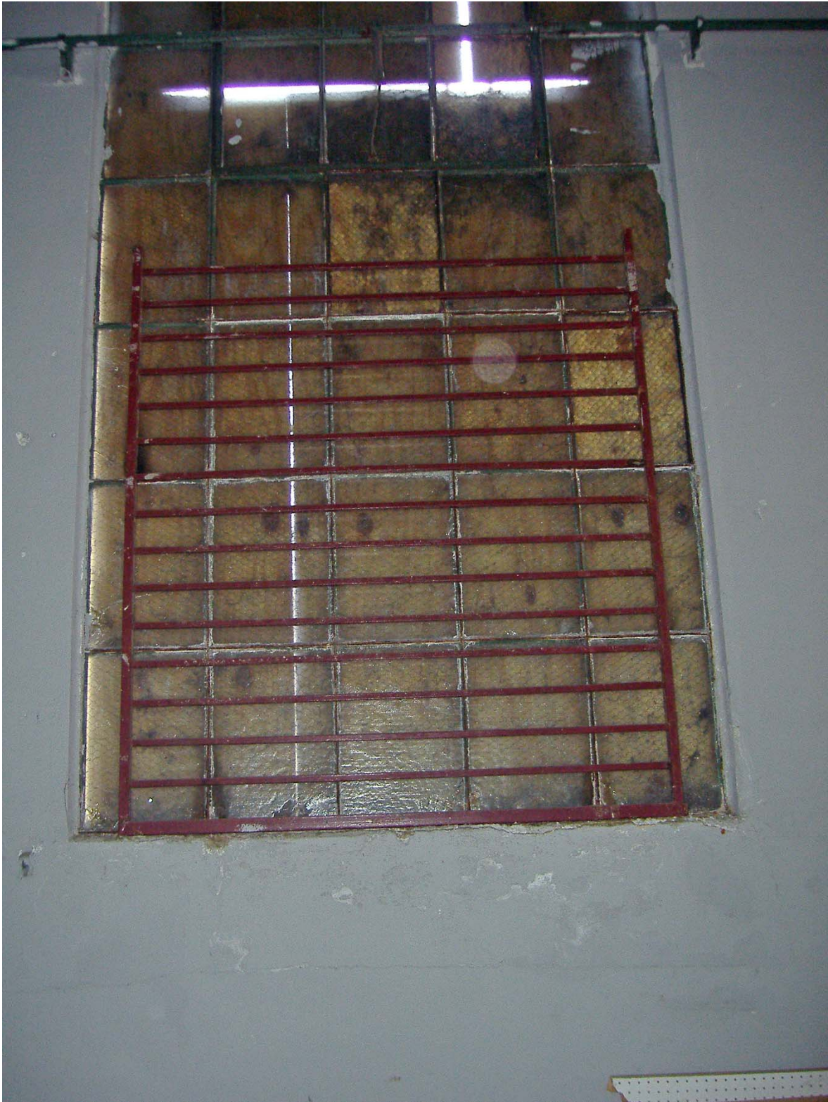
Detail of Industrial Window with Added Security Bars (West Elevation; facing West).
