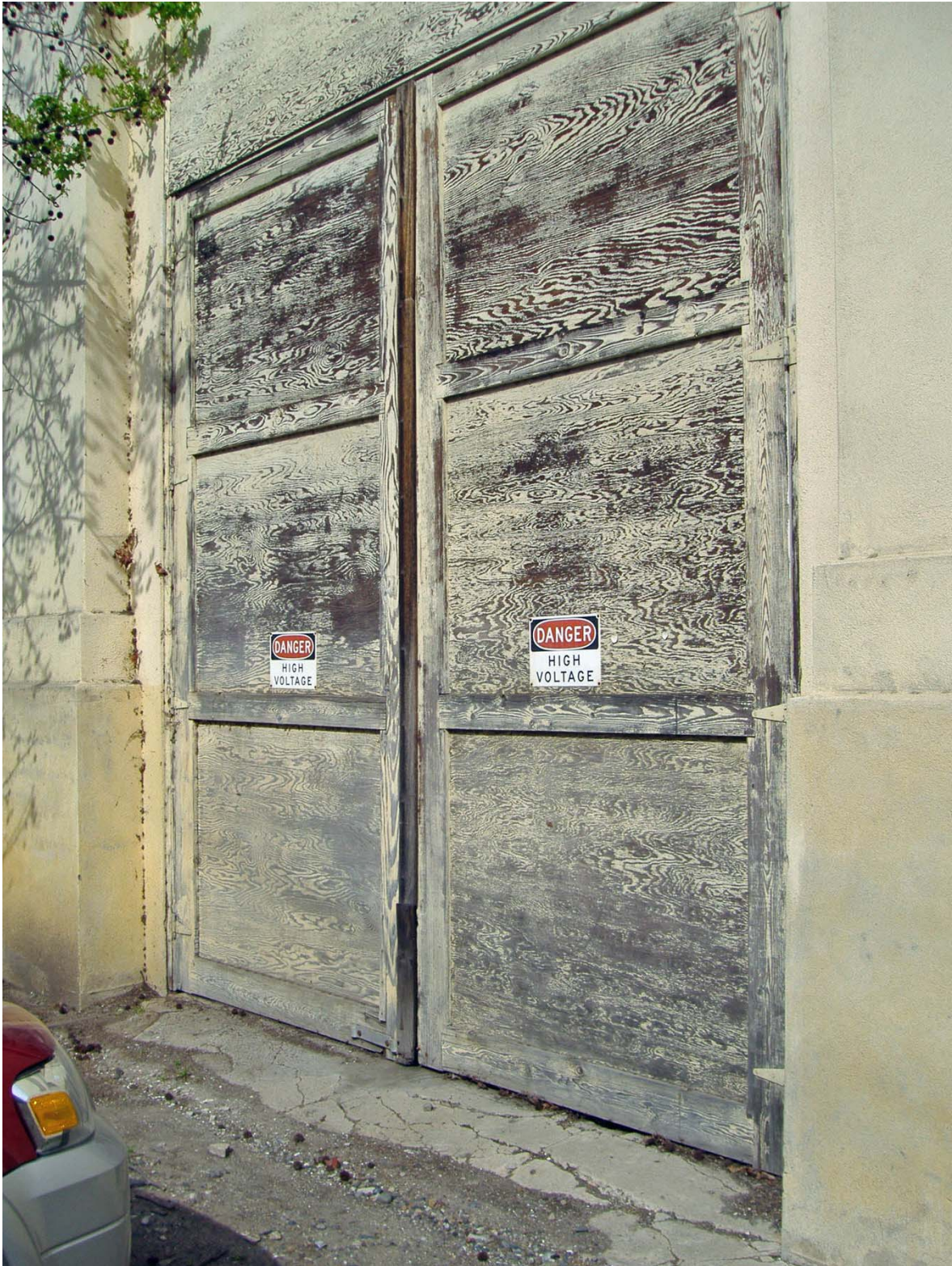
Detail of Bay Doors on South Elevation of SD G & E Building (facing Northwest).
