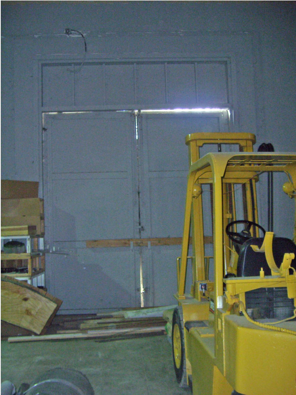
Overview of South Elevation from Interior of SD G & E Building, San Juan Capistrano (facing South).
