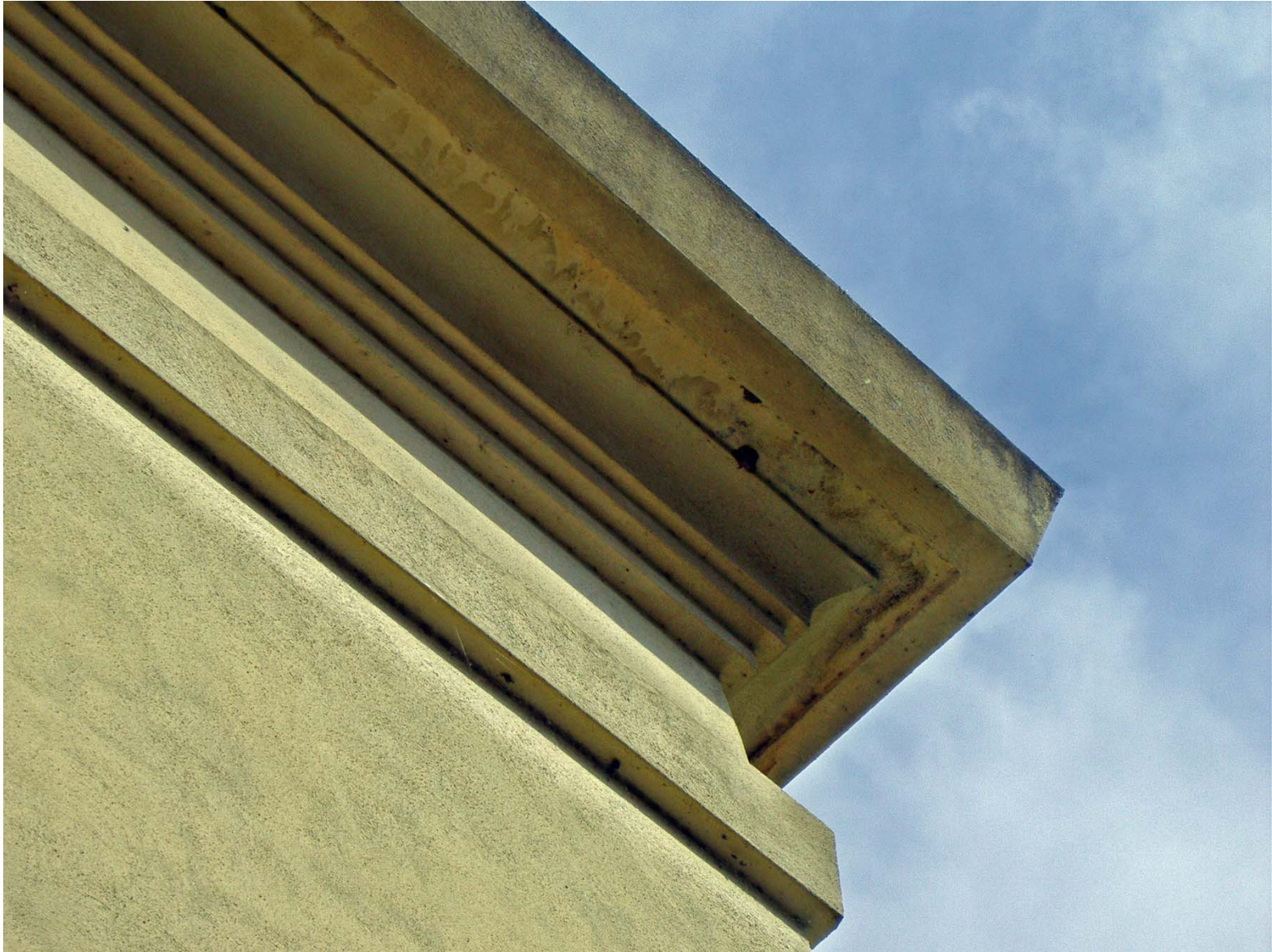
Detail fo roof Line of SD G & E Building, San Juan Capistrano (facing Northeast).
