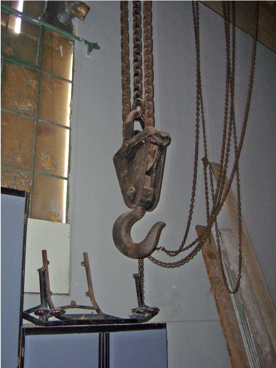
Crane Hook and Chains, SD G & E Building, San Juan Capistrano (facing Southeast).
