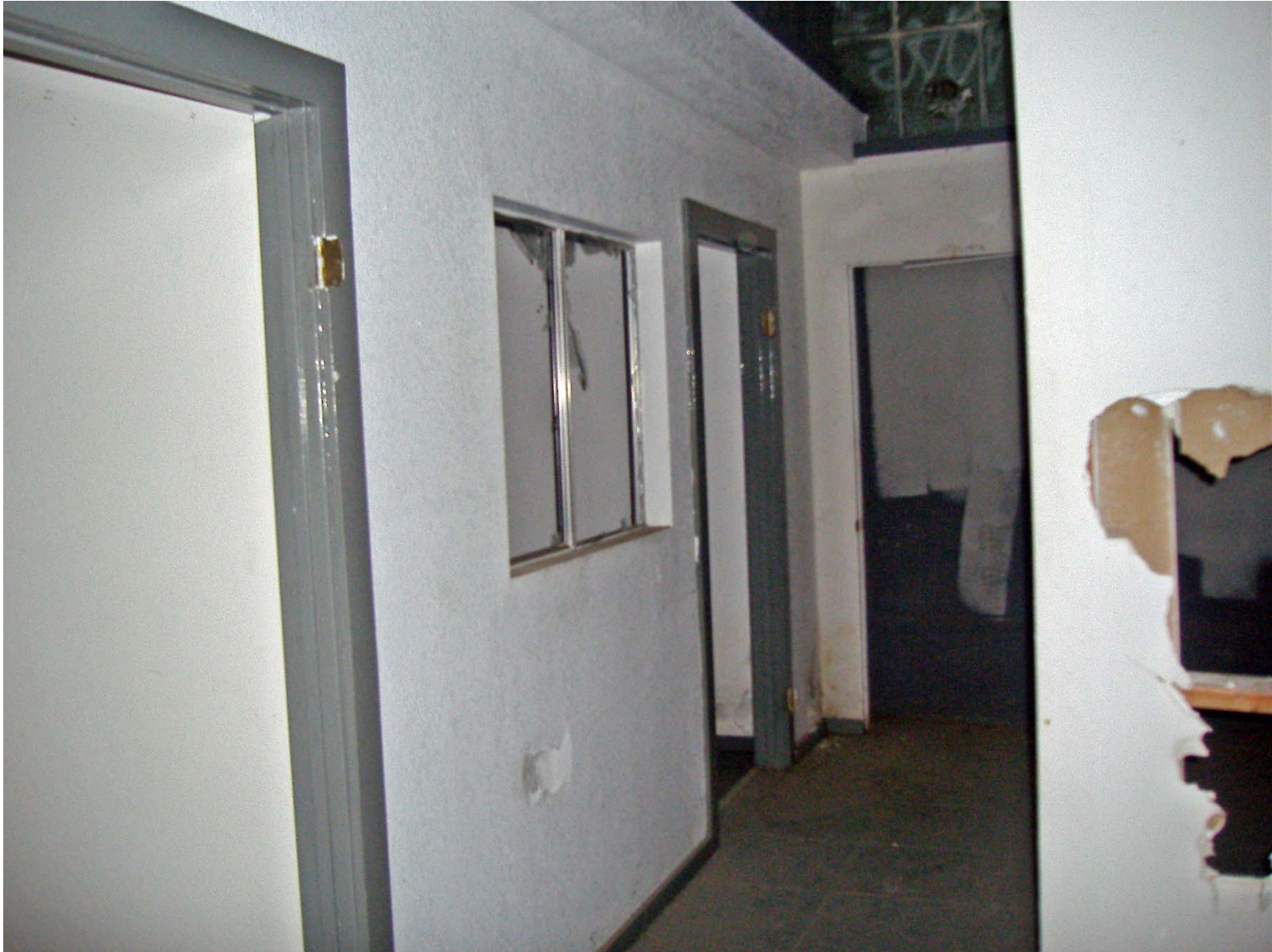
Detail of Sheet-rock Walls in Added Offices within East Ell (facing Southwest).
