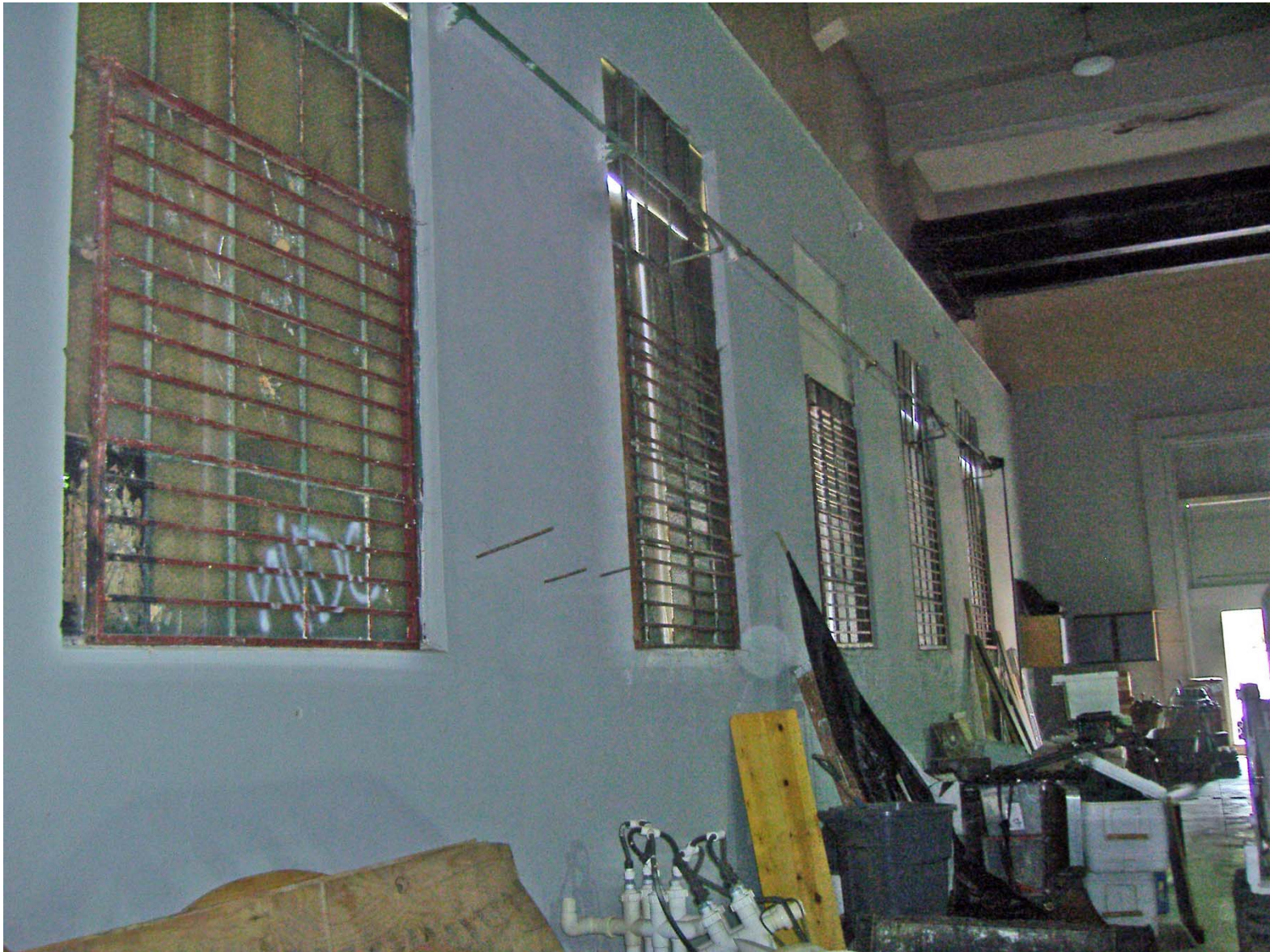
Overview of Industrial Windows on West Elevation from Interior of SD G & E Building (facing Northwest).
