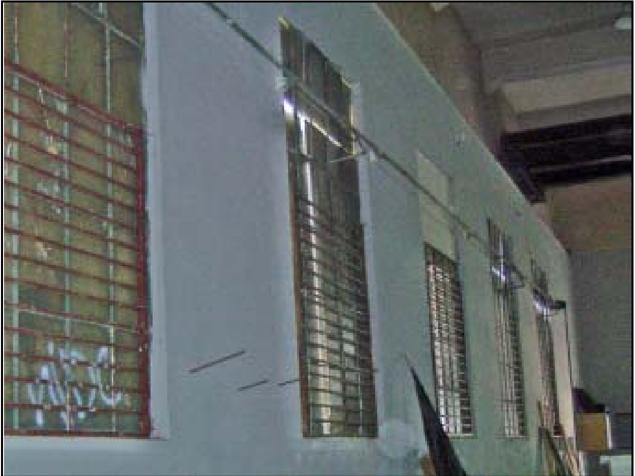
Figure 8. View of Windows on West Elevation from Interior of Structure, Illustrating the Wheel and Pulley System for Opening the Casement Windows (facing Northwest).
