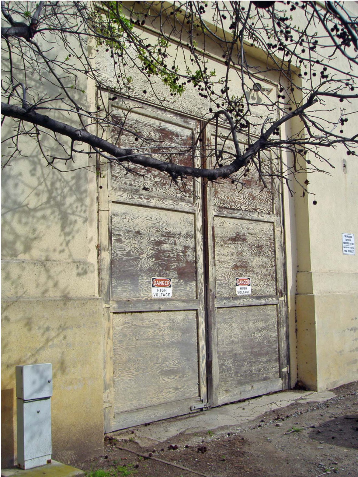
Overview of Bay Doors on South Elevation of SD G & E Building (facing Northeast).
