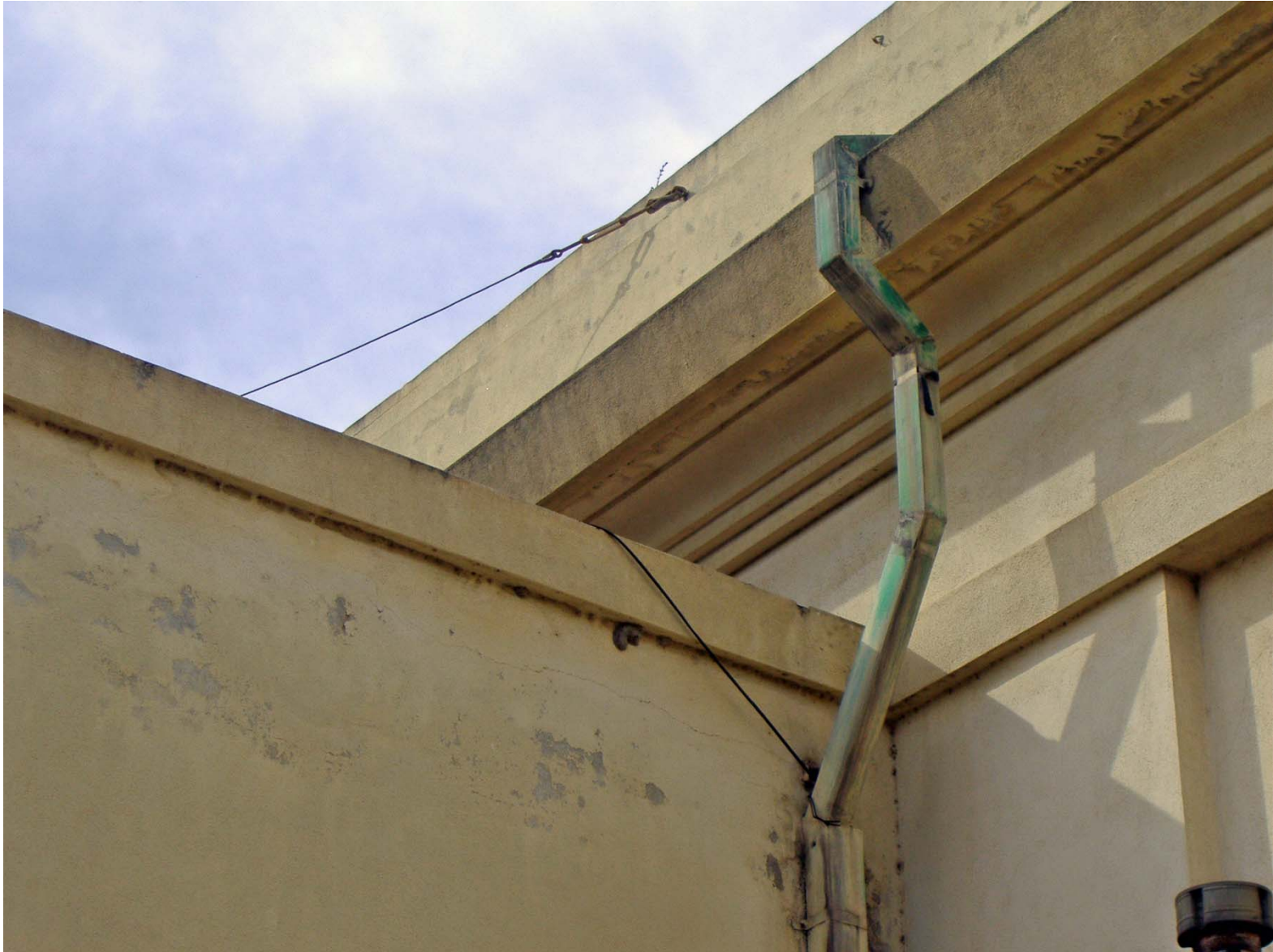
Detail of Drain Pipe and Roof Design at Corner of Main Building and East Ell, SD G & E Building (facing Southwest).
