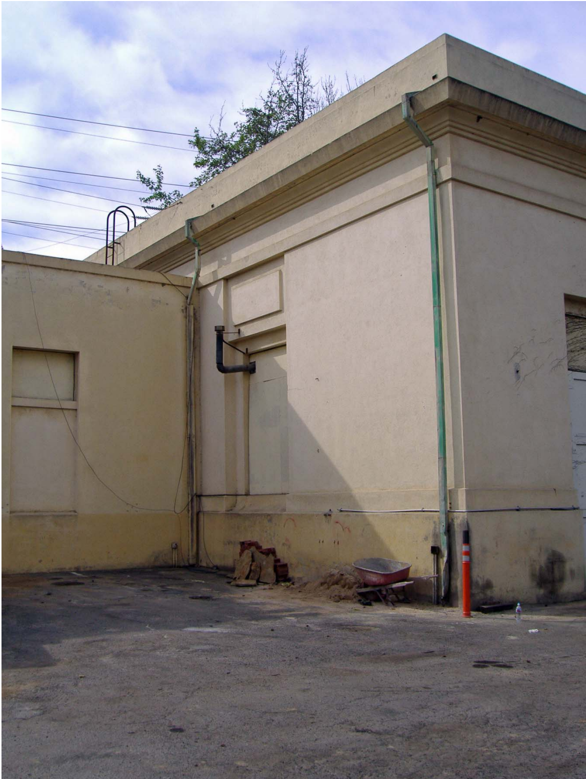
Overview of Western Portion of the SD G & E Building (facing Southwest).
