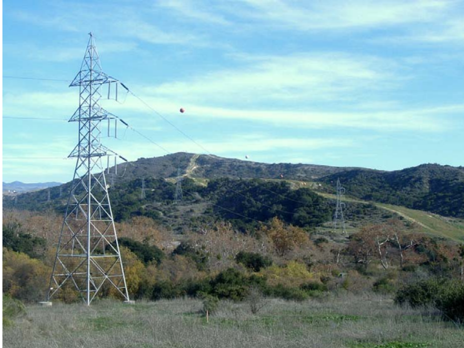
Photograph 1: Behind the Talega Substation looking north.
