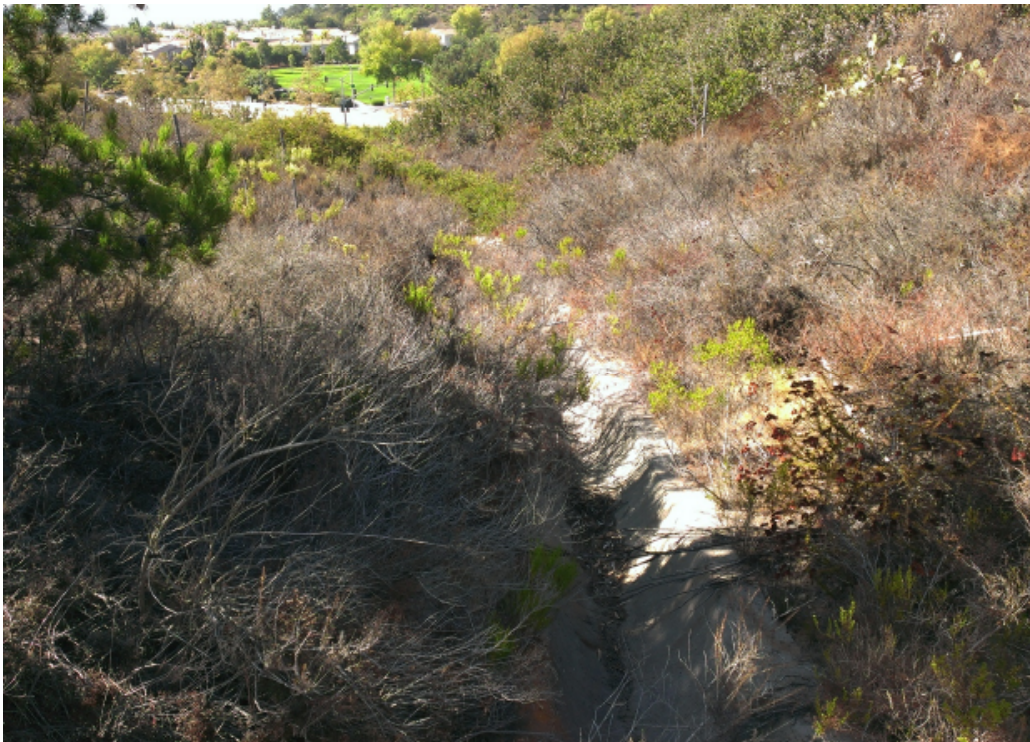
Photo 2: V-ditch draining the Peñasquitos substation pad; Photo direction: W
