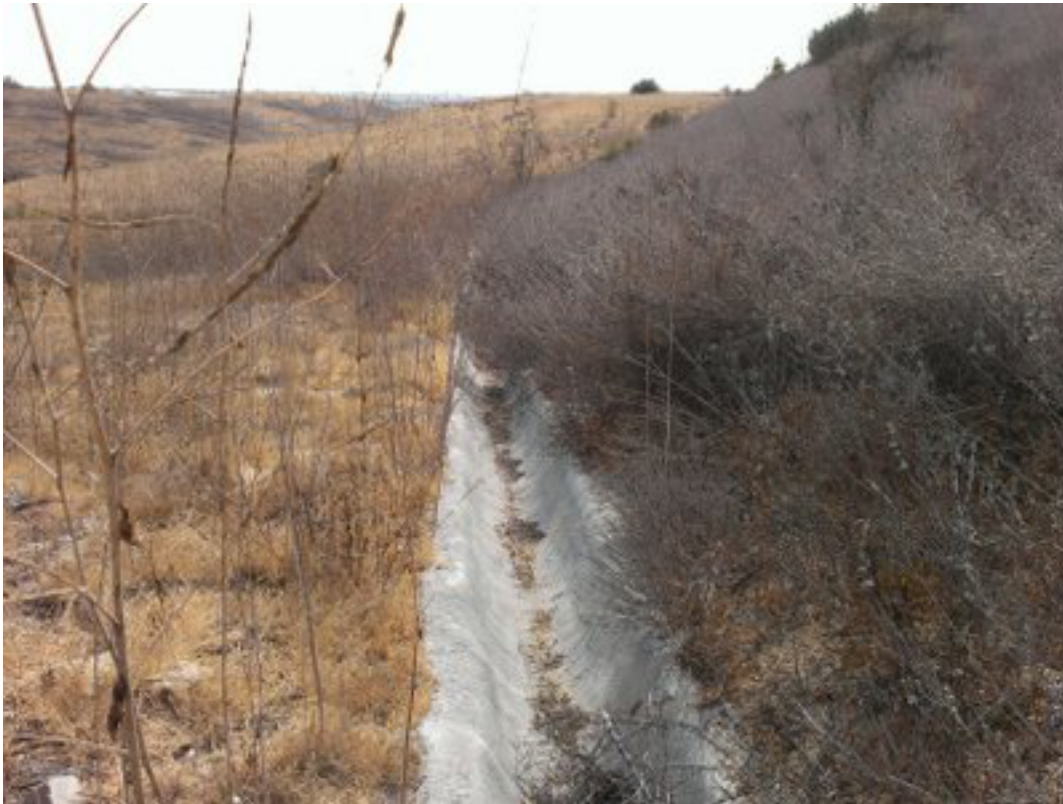
Photo 96: RWQCB exempt, MS4 erosion control V-ditch
