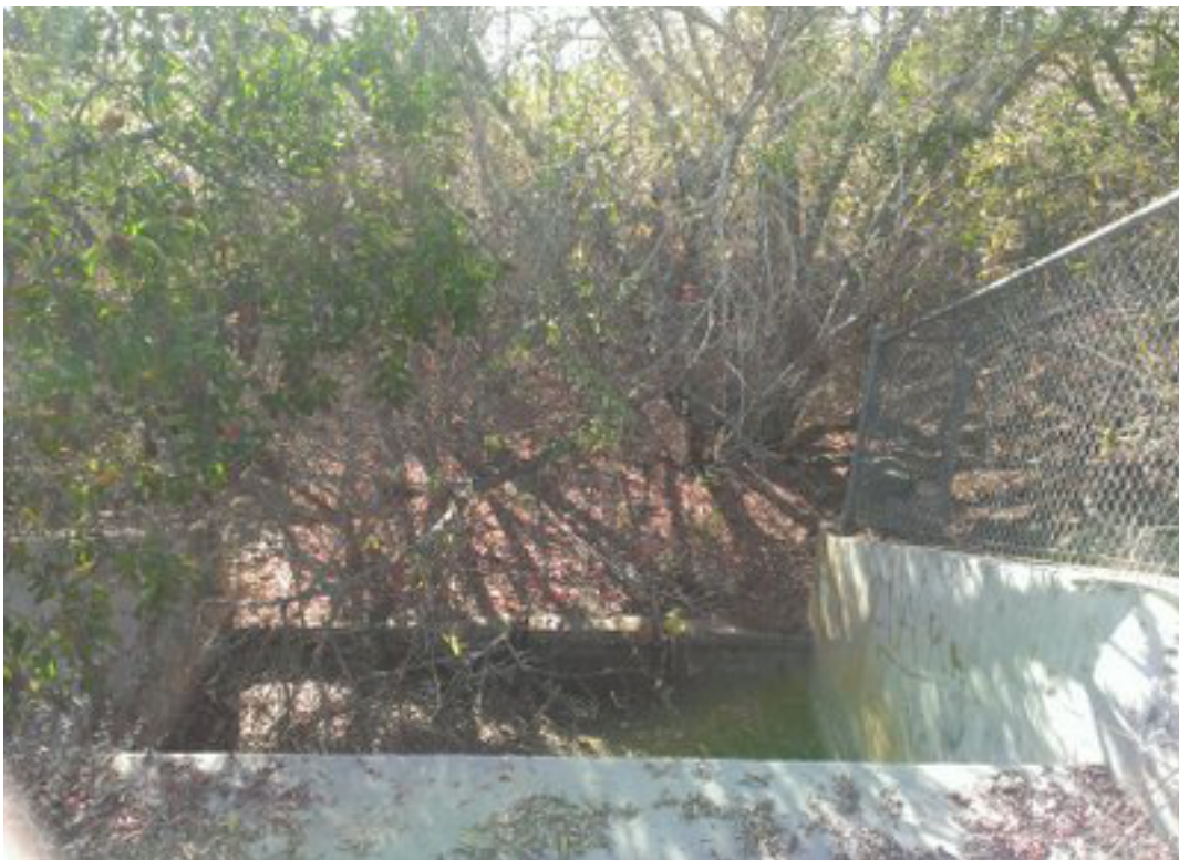
Photo 54: Tributary to La Zanja Canyon 1, culvert outlet and cobble substrate near culvert and on channel bottom
