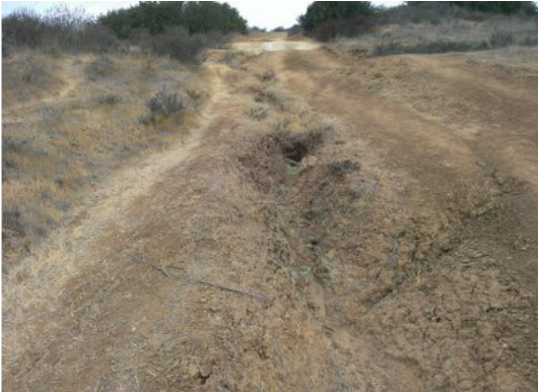
Photo 93: Vegetated road rut
