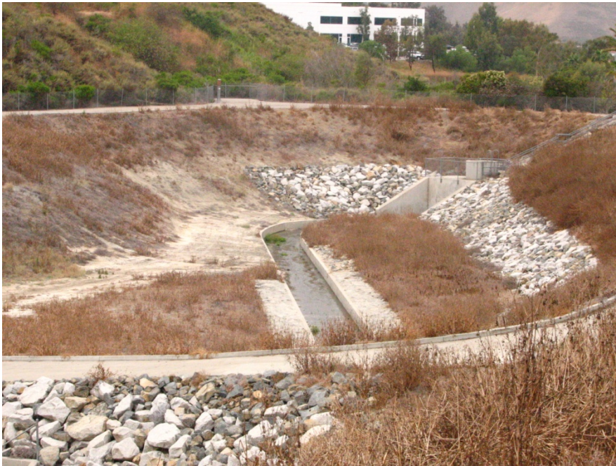
Photo 12: View of Tributary Segunda Deshecha Cañada 2 facing west. The tributary is a maintained flood control facility.
