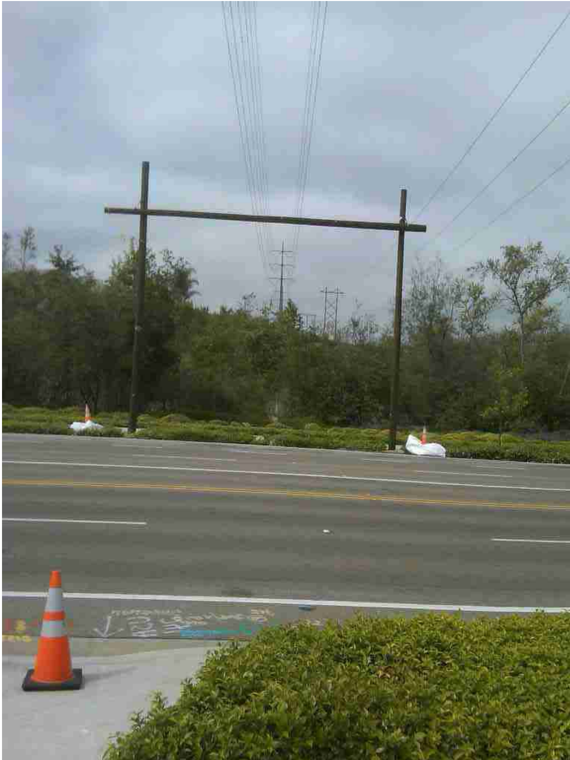
Typical wood guard structure at a road crossing
