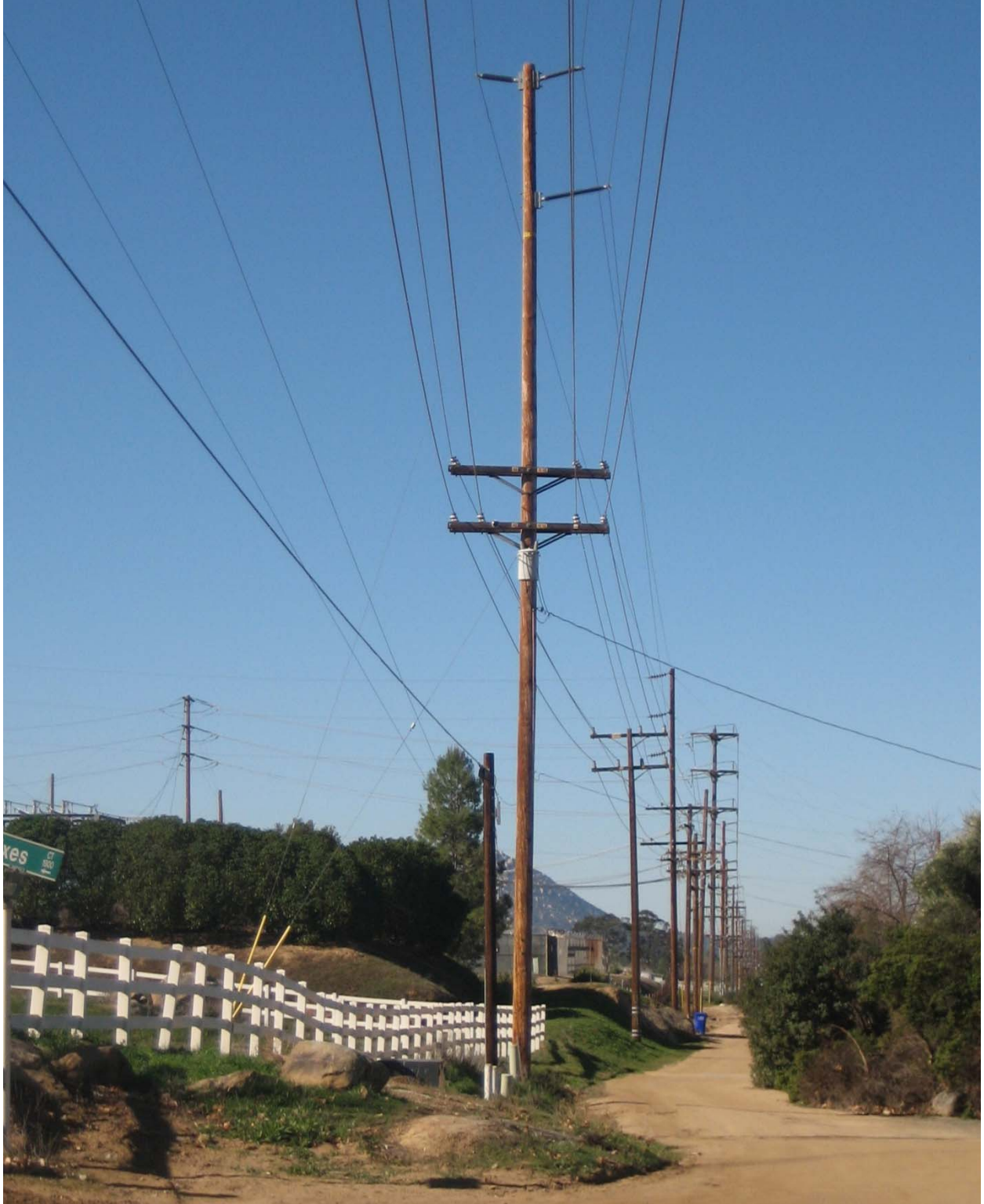
Typical wood transmission pole (with distribution underbuild)
