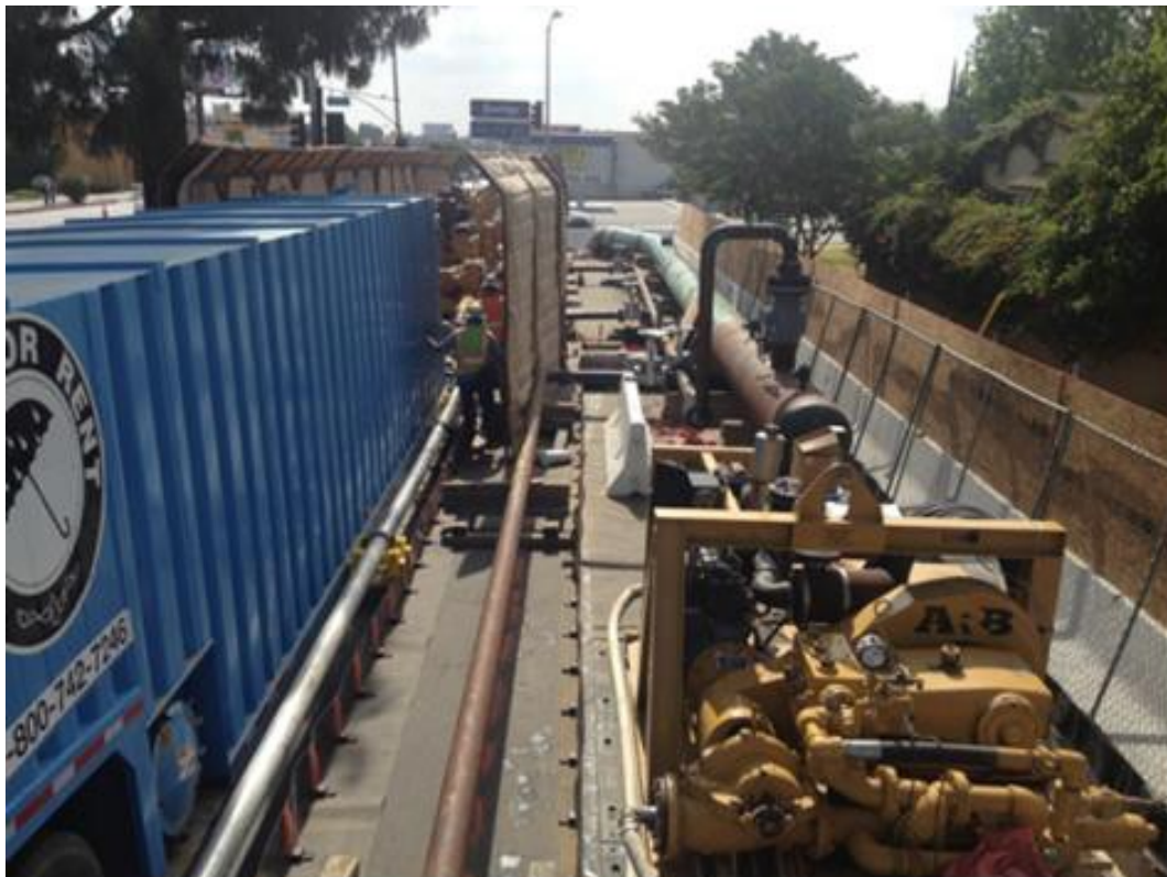
Figure 11: Hydrotest Set Up with Sound Proofing to Minimize Noise Complaints (located behind Baker tank)
