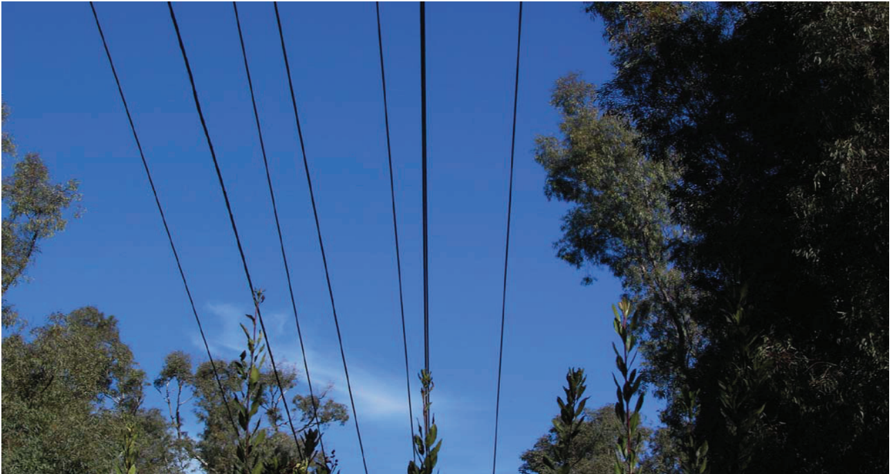
Figure 12: Reliability trees may not always be readily observable. In the example below, the tall, slender eucalyptus tree has a slight lean and may be well clear of the electrical facilities during normal weather conditions.
