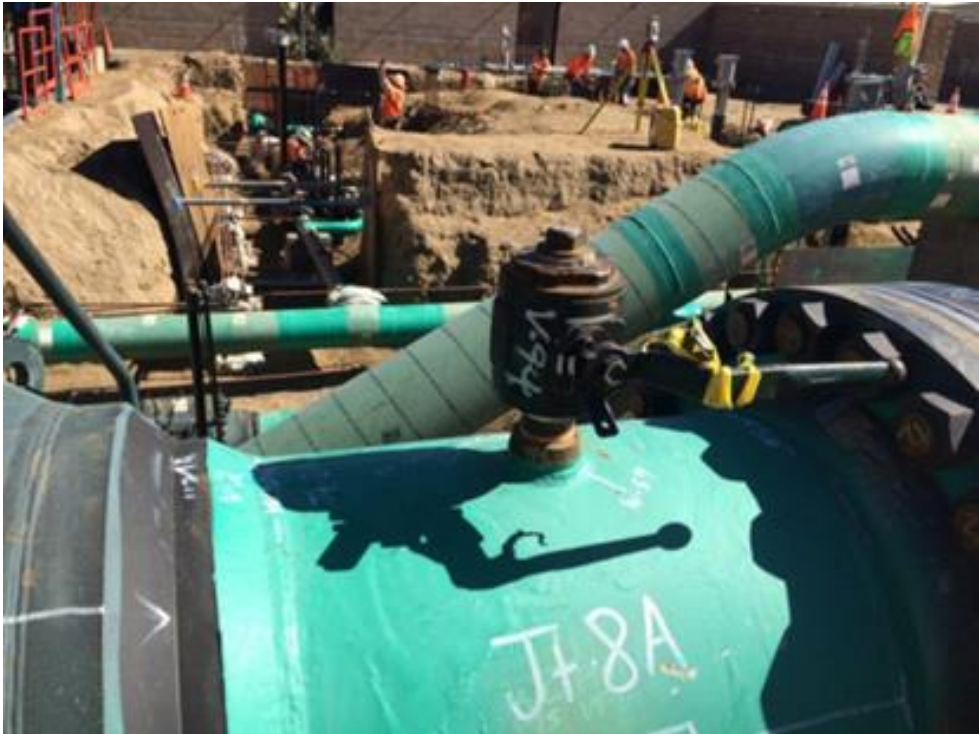
Figure 18: Large Valve Station with Numerous Above-Ground Features
