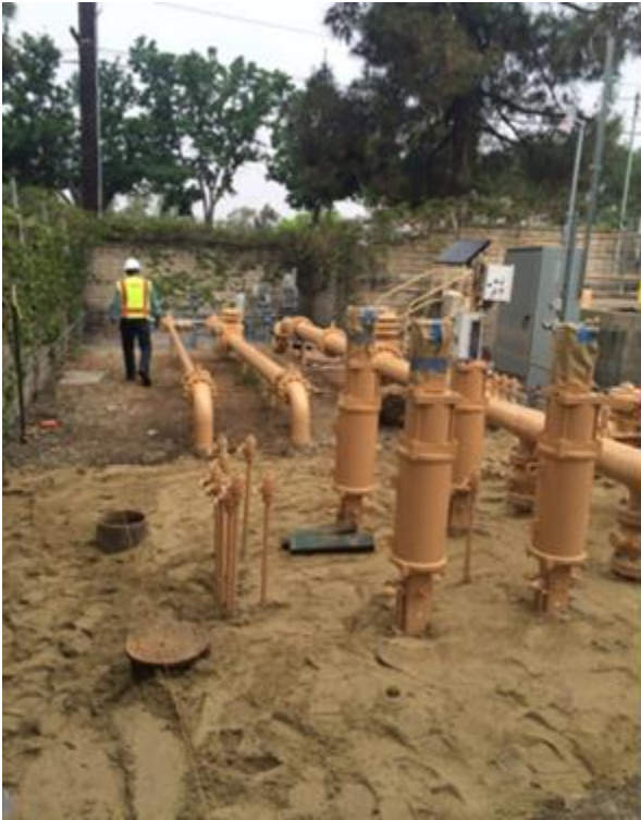
Figure 17: Above-Ground Valve Equipment
